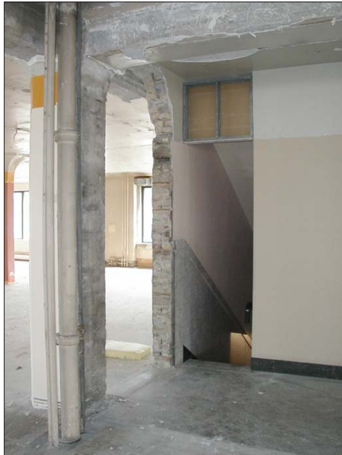
Plate 10 – Canada Building, fourth floor. ( M. Peterson, 2003. )
