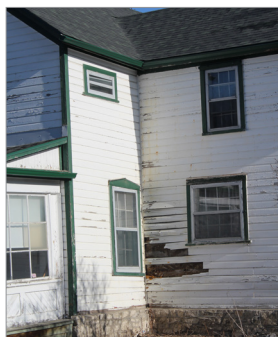
Bleak House, 1637 Main St., showing deteriorated original wood siding, 2025
