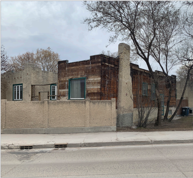
Unit 1, 40 St. Mary’s Rd., stucco removed, 2024
