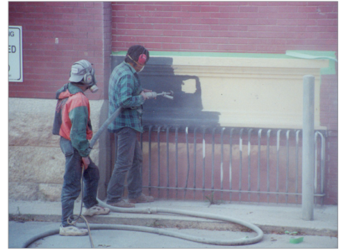
Customs Examining Warehouse, 145 McDermot Ave., sand blasting the metal to remove paint, 2000
