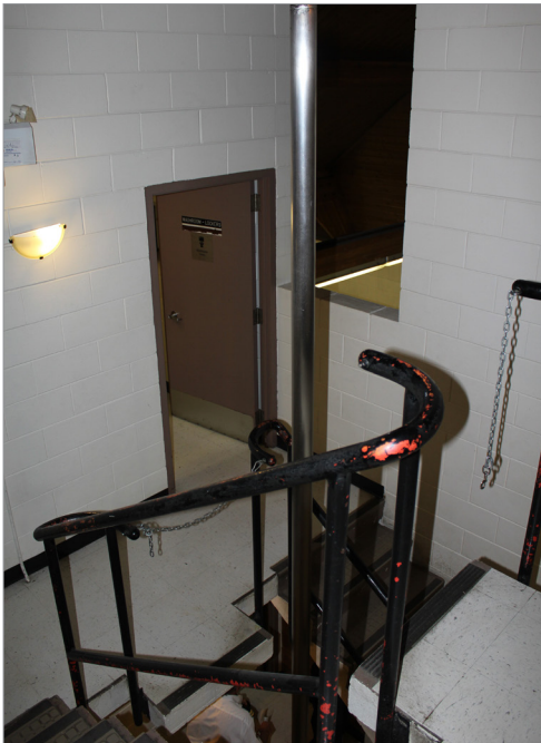
Fire Station No. 4, 1083 Autumnwood Dr., stairs and firefighters' pole, 2021
