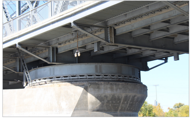
Redwood Bridge, swing span machinery, 2022
