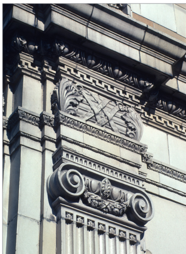
Terra cotta ornamentation on the Lindsay Building, 228 Notre Dame Ave., 1980
