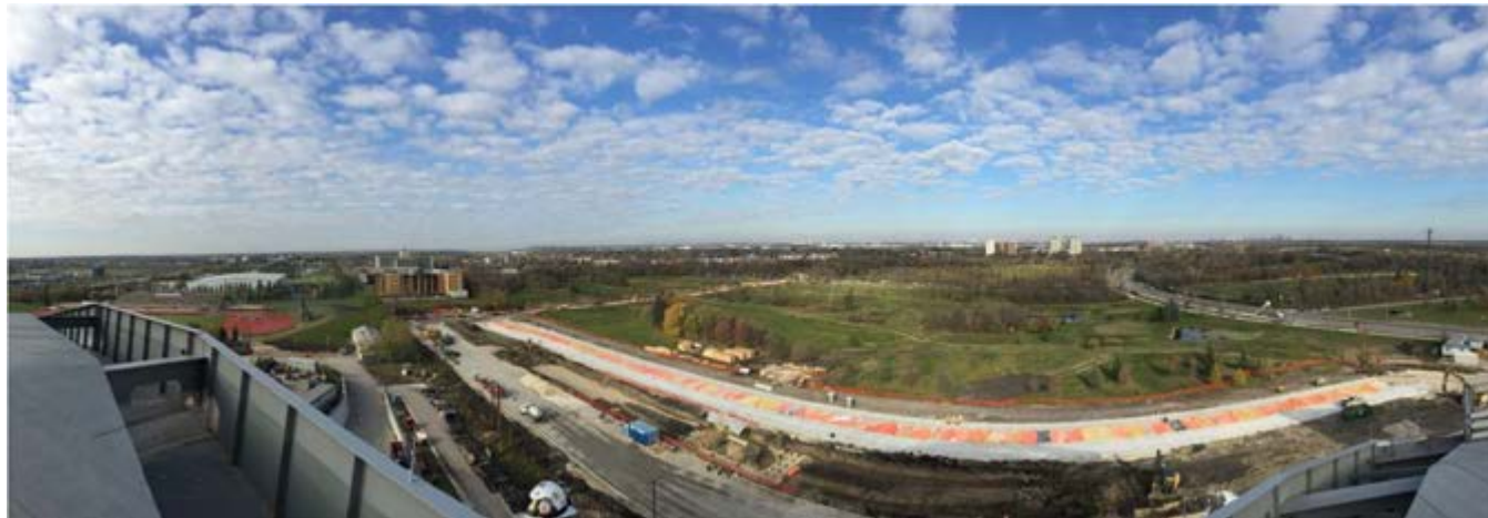
Overhead view of Southwest Rapid Transitway construction linking to Investors Group Field / University of Manitoba
