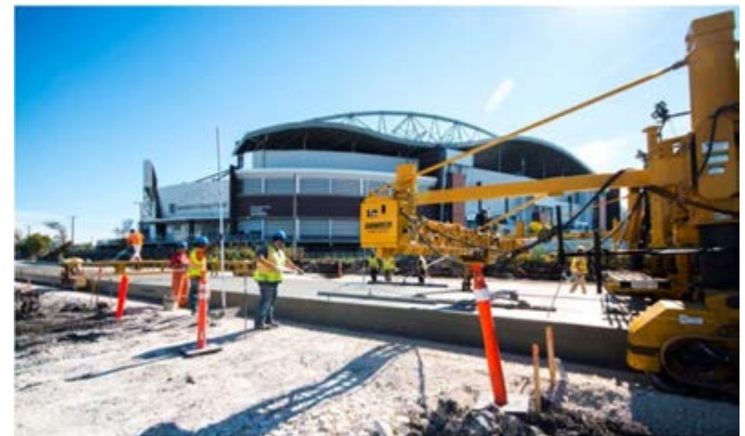
Construction of Southwest Rapid Transitway at Investors Group Field / University of Manitoba
