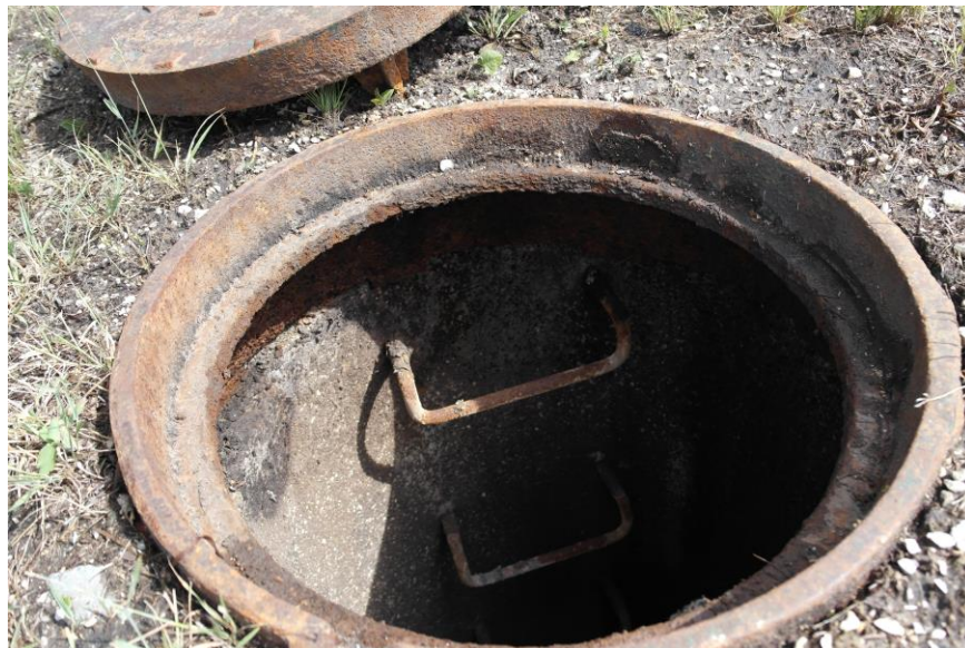
Riverbend Lift Station Wet Well
