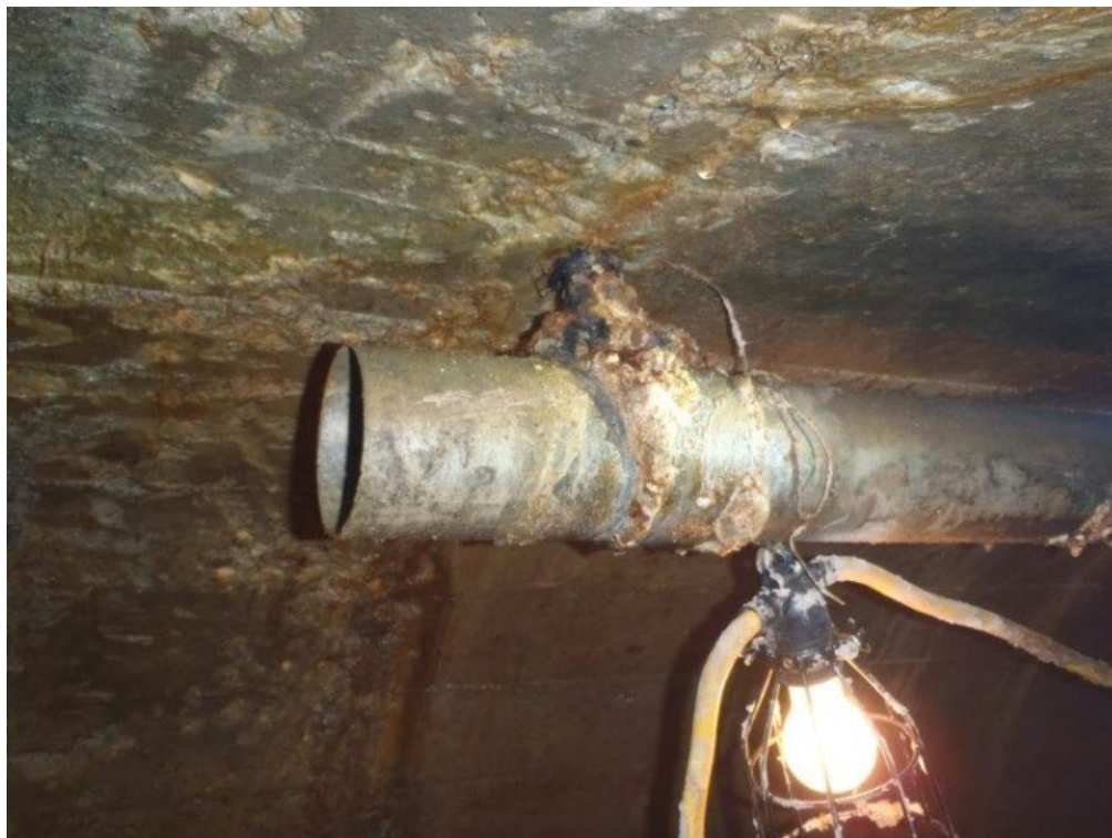
West Side – Existing tunnel ventilation piping (typ)
