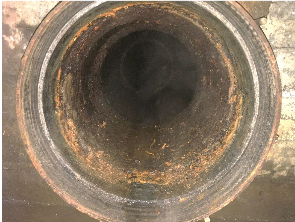
East Side - 600 feeder main (interior)
