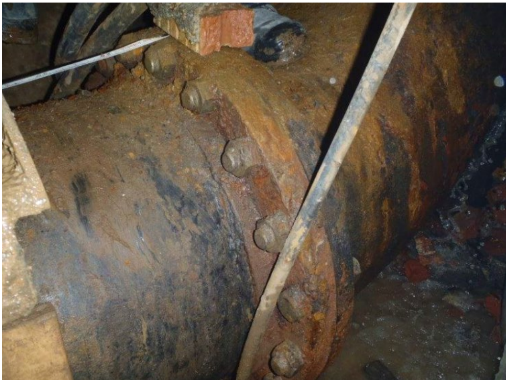
West Side – Existing 600 mm feeder main lower 90 deg bend lower flange connection
