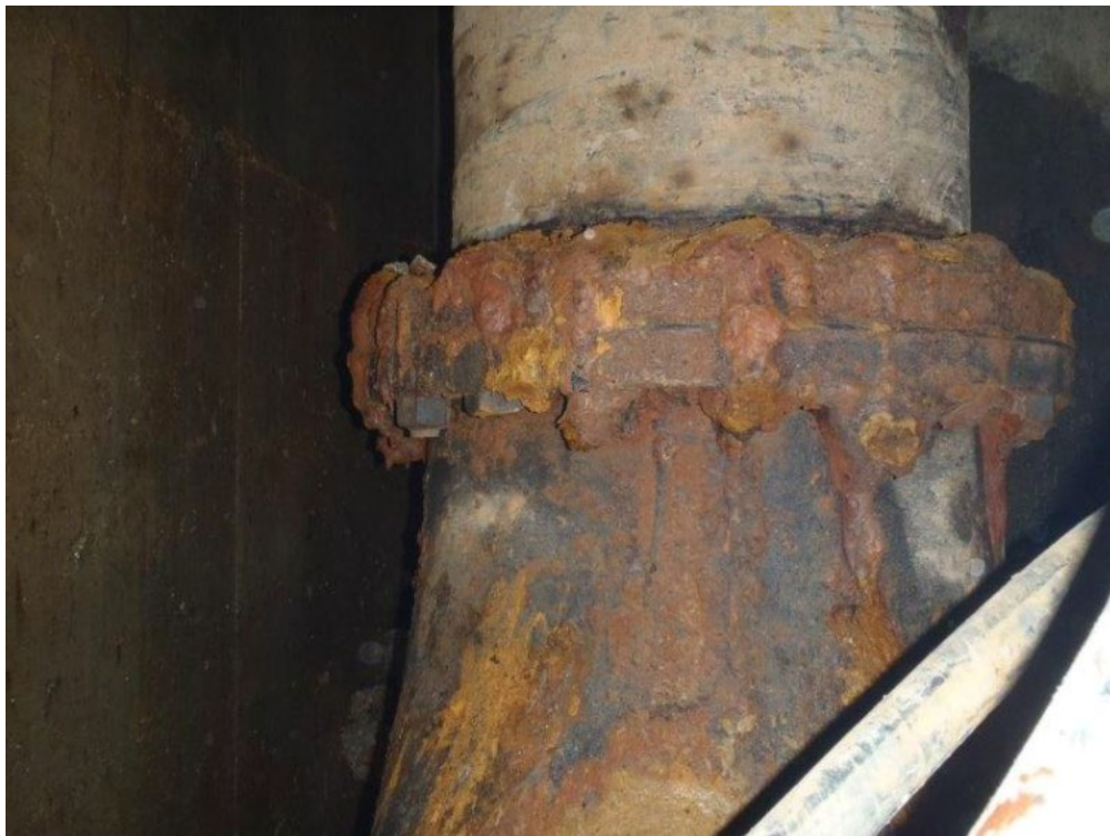
West Side – Existing 600 mm feeder main lower 90 deg bend upper flange connection
