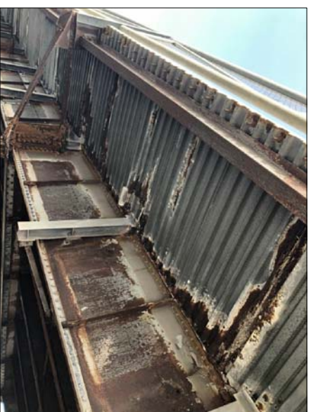
EXISTING CONDITION OF CORRUGATED STEEL DECKING UNDER SIDEWALK
