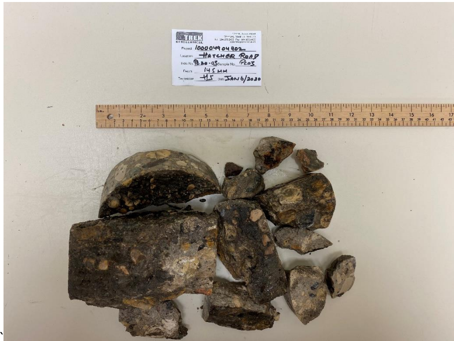
Photo 3: Pavement Core Sample at Pavement Hole at JOINT PC20-03
