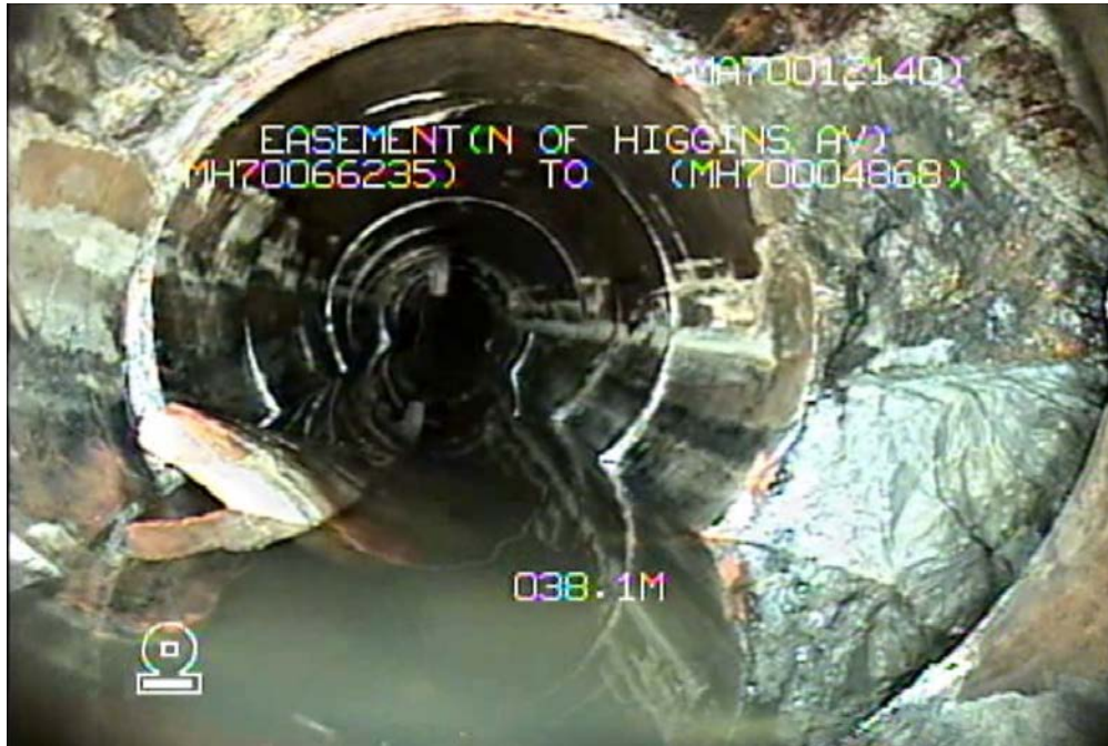
Figure 5 – Sheet 4, Dwg 12268, S-MA70012140 (Easement N. of Higgins) – Hole with Debris at 38.0m upstream of MH70066235
