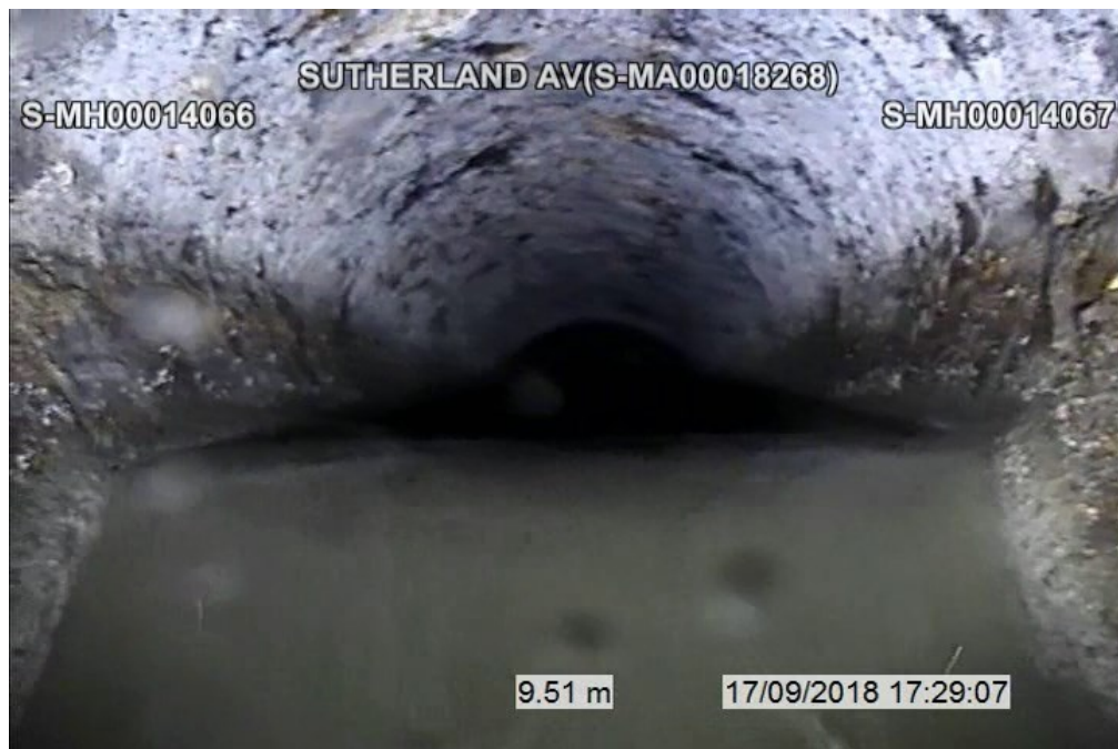
Figure 16 – Sheet 23, Dwg 12287, S-MA00018268 (Sutherland Av.) – Stepped Diameter Change from 900 mm to 1100 mm at 10.1m Downstream.
