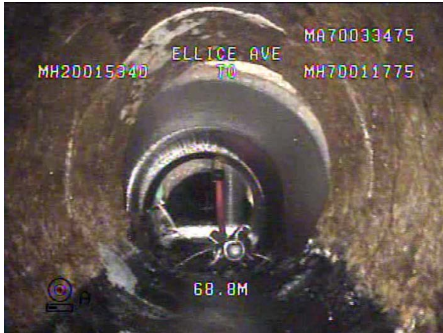
Figure 9 – Sheet 8, Dwg 12272, S-MA70033475 (Ellice Av.) – Material and Cross Section Change to Circular Vitrified Clay.
