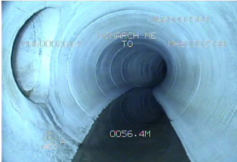
Figure 15 – Sheet 15, Dwg 12279, S-MA60003590 (Vialoux Dr.) – Downstream Tee Connection as Seen from Asset S-MA60003569.
