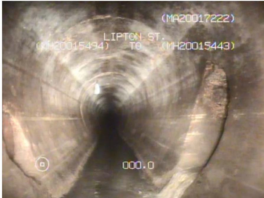
Figure 13 – Sheet 6, Dwg 12270, S-MA20017229 (Ellice Av.) – Downstream Tee Connection on Lipton St as Seen from Asset S-MA20017222.
