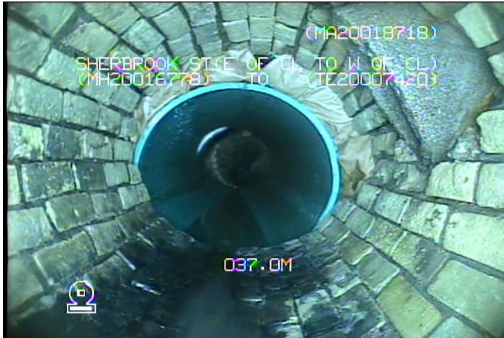
Figure 23 - Sheet 05, Dwg 12269, S-MA20018718 (Sherbrook St) - PVC Repair at 38.0 - 41.8 m Downstream
