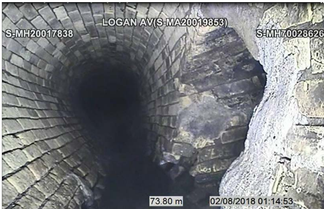
Figure 6 – Sheet 5, Dwg 12269, S-MA20018718 (Sherbrook St.) – Downstream Tee Connection on Logan Av as Seen from Asset S-MA20019853.
