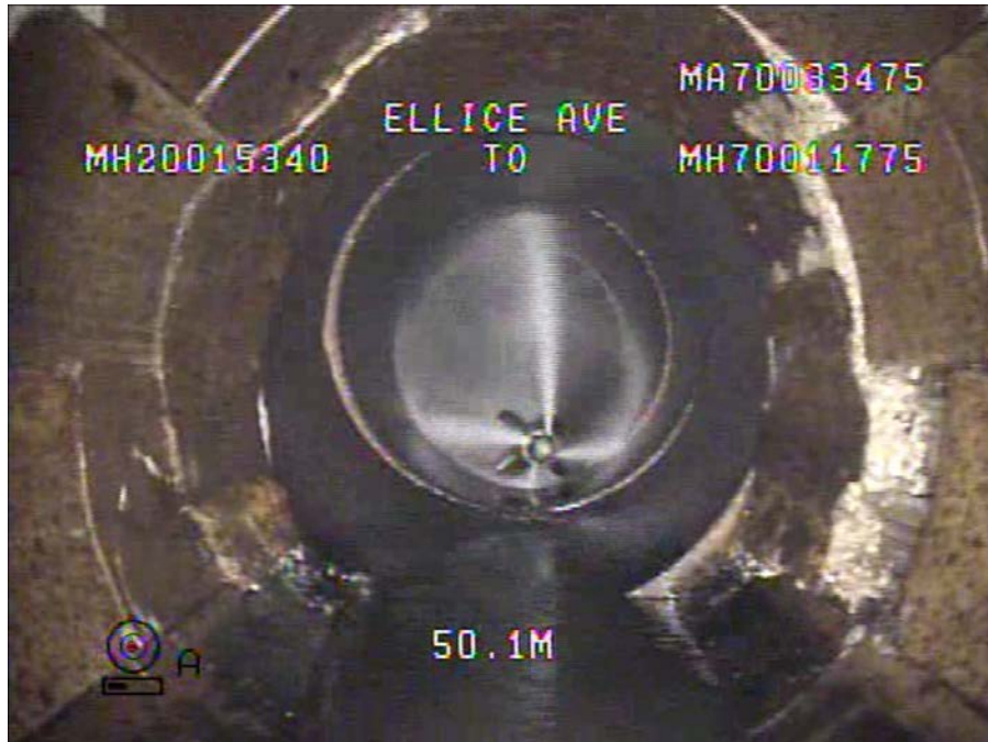
Figure 7 – Sheet 8, Dwg 12272, S-MA70033475 (Ellice Av.) – Material Change from Segmental Clay Tile to Vitrified Clay at 50.8 m Downstream.
