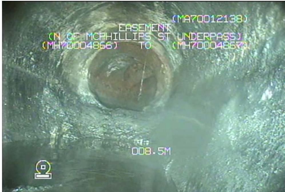
Figure 1 – Sheet 3, Dwg 12267, S-MA70012138 (McPhillips St) – Transition from 1100 mm Egg Sewer to 600 mm Fabricated Steel Elbow upstream of MH70004867.
