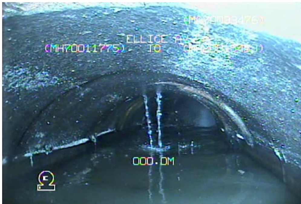
Figure 10 – Sheet 7, Dwg 12271, S-MA70033476 (Ellice Av.) – Infiltration (Gusher) at 3.0 m Downstream.
