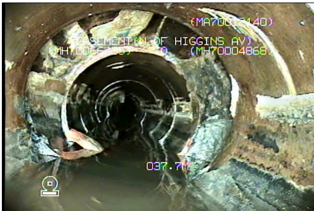
Figure 4 - Sheet 4, Dwg 12268, S-MA70012140 (Easement N. of Higgins) – Hole with Debris at 38.0m upstream of MH70066235
