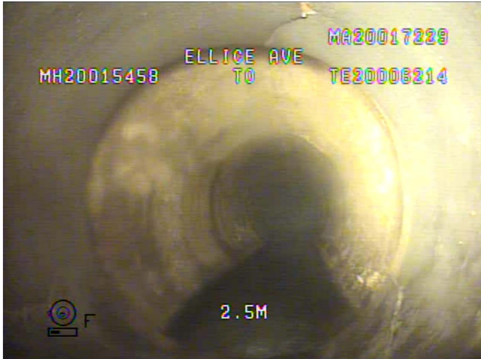
Figure 11 – Sheet 6, Dwg 12270, S-MA20017229 (Ellice Av.) – Apparent Diameter Change from 750 mm to 900 mm at 3.0 m Downstream.
