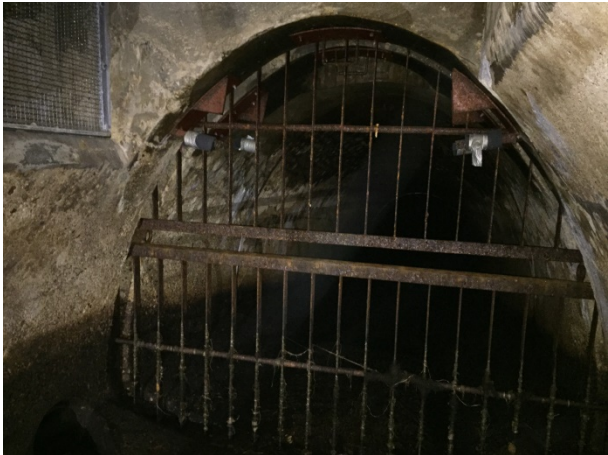
Photograph 8. ↑ Mile 17.05 – Existing Groove (Grating to be Removed)
