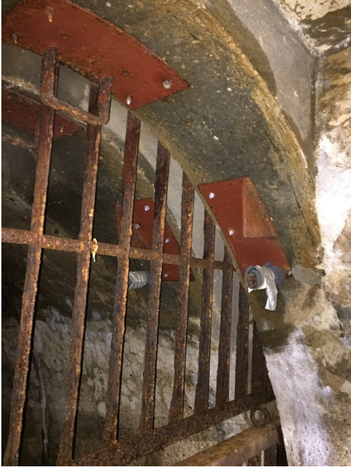
Photograph 6. ↑ Mile 17.05 – Existing Groove (Grating to be Removed)
