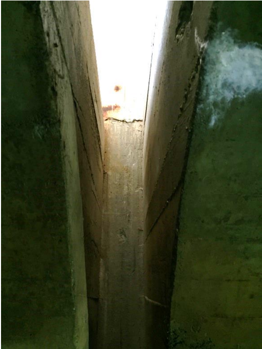
Photograph 22. ↑ Mile 73.69 – Existing Groove (Top Corner, Below Floor Opening)
