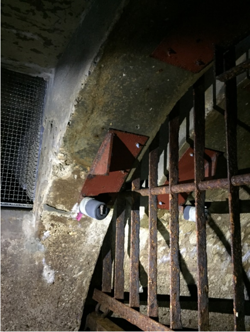
Photograph 5. ↑ Mile 17.05 – Existing Groove (Grating to be Removed)
