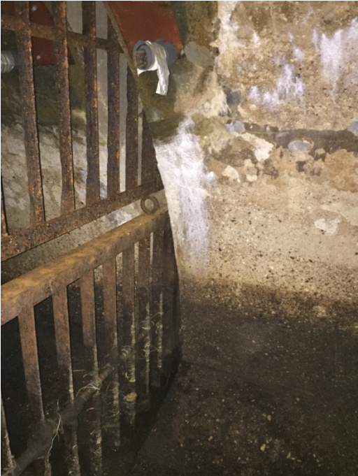
Photograph 7. ↑ Mile 17.05 – Existing Groove (Grating to be Removed)
