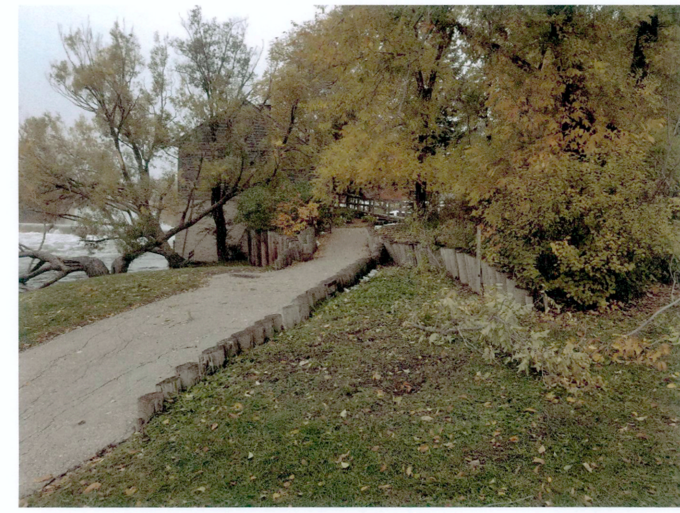
PHOTO 'A' (TO BE REMOVED AND REPLACED)
