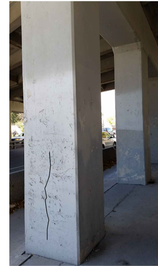
2. EAST AND NORTH FACE COLUMN 14 (LINE ADDED TO ILLUSTRATE CRACK LOCATION)
