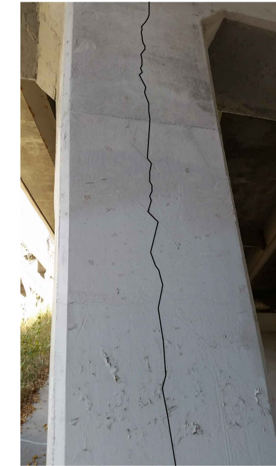
1. SOUTH FACE COLUMN 11 (LINE ADDED TO ILLUSTRATE CRACK LOCATION)
