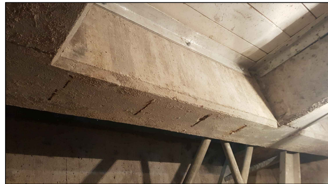
RUSTED STIRRUPS IN CONCRETE BEAM IN COMMUNOTOR FLOOR
