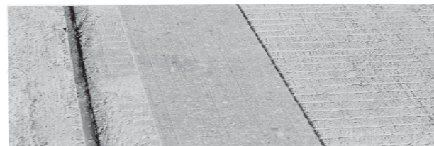
Figure 8 – PCC Light Corduroy or ribbed pattern made with properly spaced, gang stacked cutting blades.
