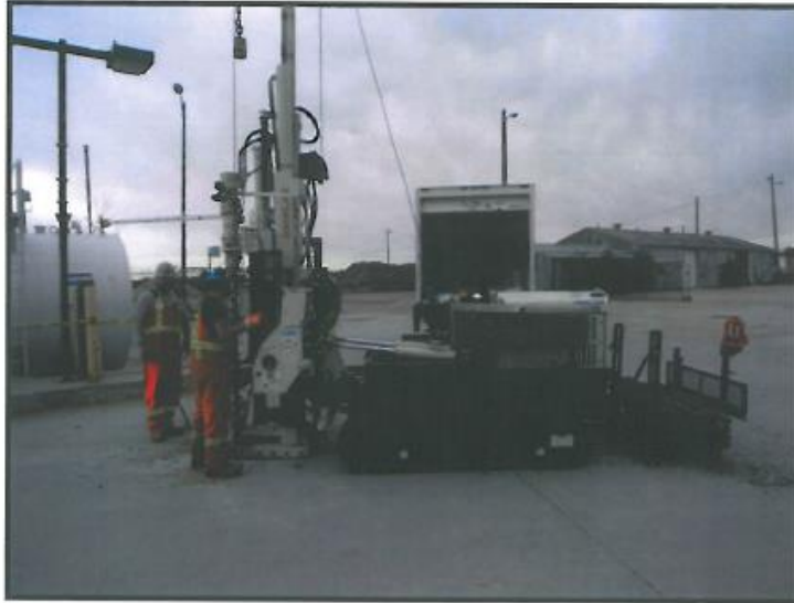
PHOTOGRAPH #1: Site, facing southeast showing the drilling of TH1 near the abandoned AST's on 849 Ravelston Avenue. In the background Commercial Building C of 1500 Plessis Road to the southeast.
