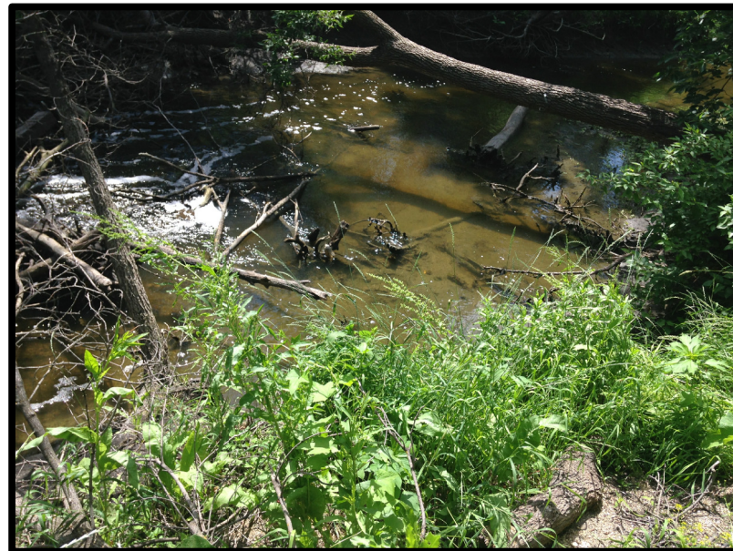
PHOTOGRAPH 10: ZONE H, FACING SOUTH, SHOWING STEEP INCLINE FROM TOP OF BANK (PATHWAY) TO CREEK SHORELINE AT FAILED REGION.
