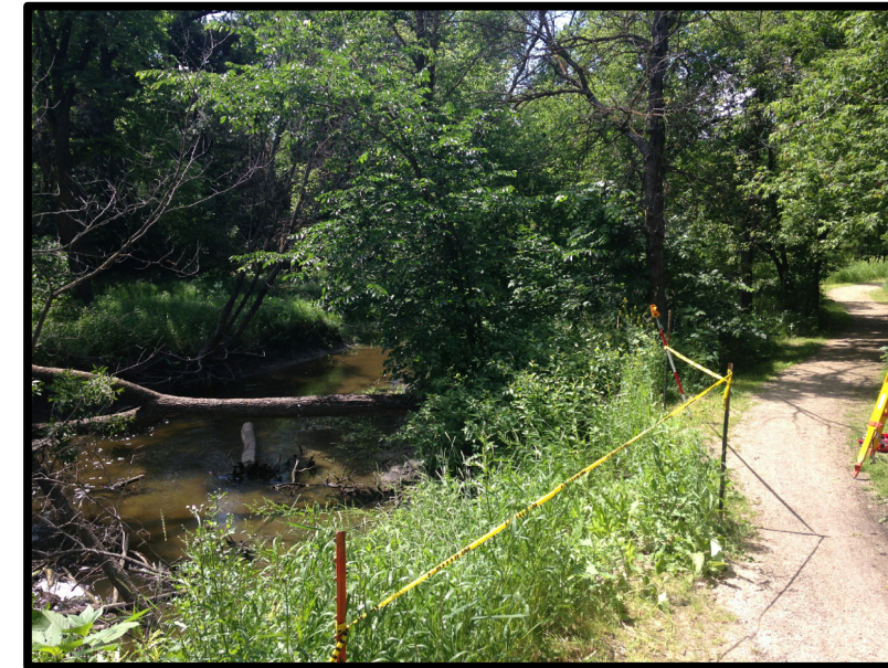
PHOTOGRAPH 9: ZONE H, FACING WEST, SHOWING FAILED REGION AT TOP OF BANK.
