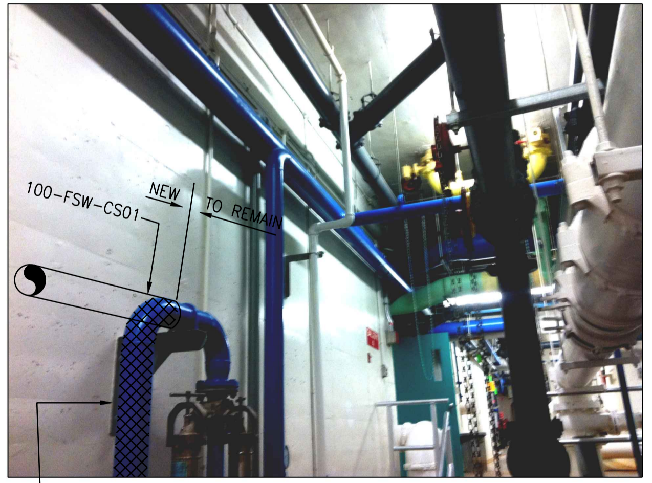
1 PHOTO REMOVE 100-FSW-CS01 AS INDICATED CLEAN AND PREP SURFACE WELD AND REROUTE AS SHOWN
