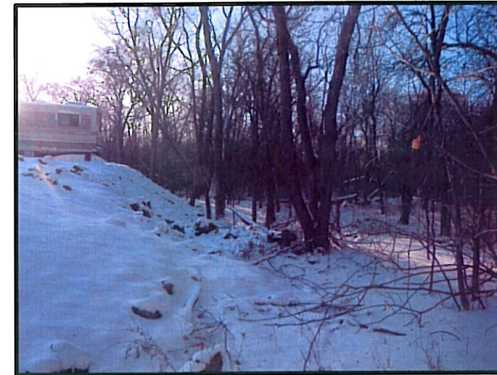
PHOTOGRAPH #6: FACING NORTHWEST, SHOWING GRADE OF SIDE SLOPES OF THE NORTH SIDE OF EXISTING BERM.
