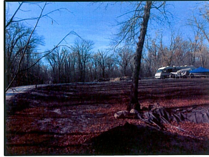
PHOTOGRAPH #2: FACING WEST, SHOWING CONSTRUCTED FLOOD PROTECTION BERM PRE HOUSE RELOCATION ALONG DRIVEWAY NEAR SOUTH PROPERTY LINE
