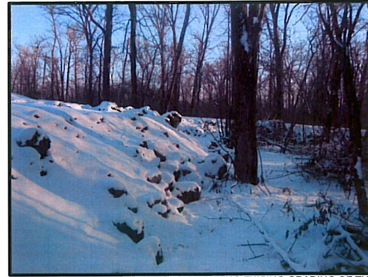
PHOTOGRAPH #8: FACING SOUTH, SHOWING EXISING GRADING OF THE WEST SIDE OF THE EXISTING BERM.
