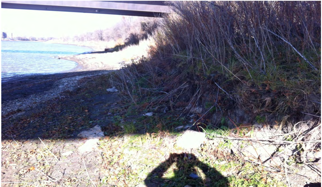
Photo 6: Erosion of riverbank toe, facing north.
