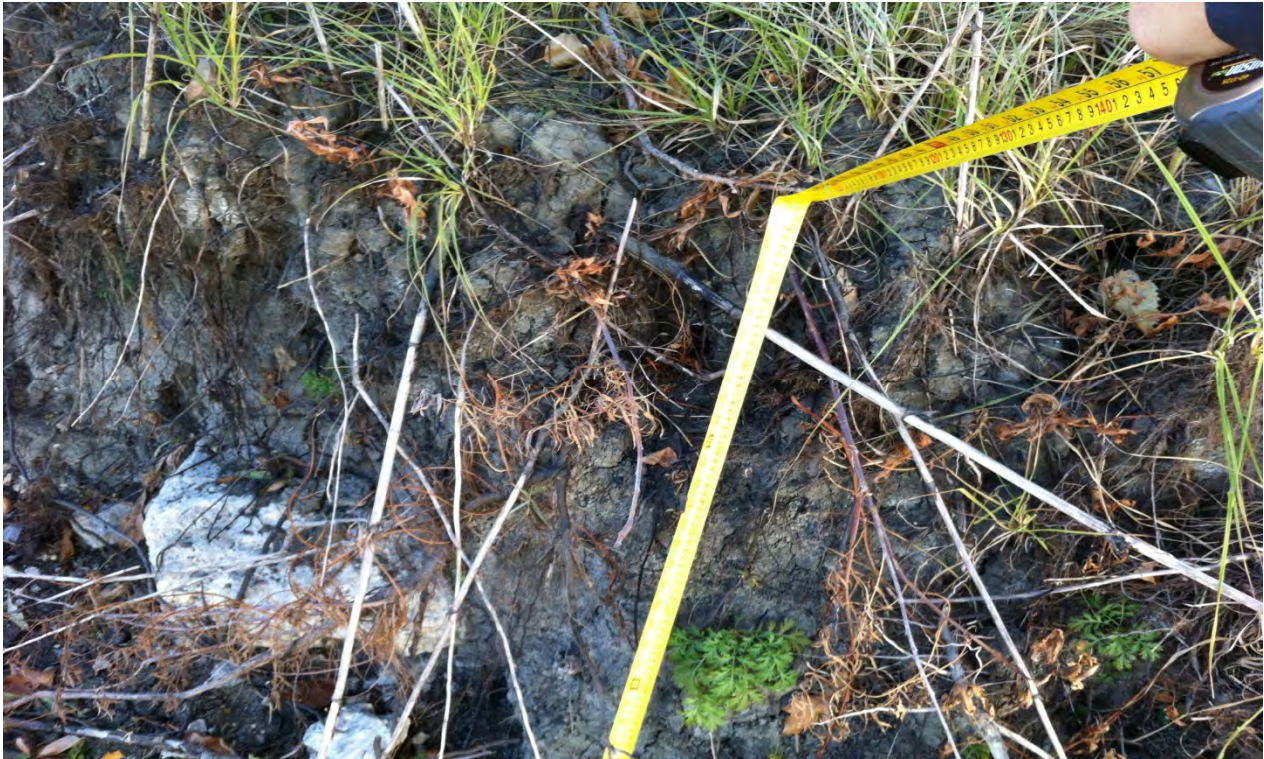
Photo 3: Exposed alluvial soils within eroded riverbank toe (highly weathered and softened), facing east.
