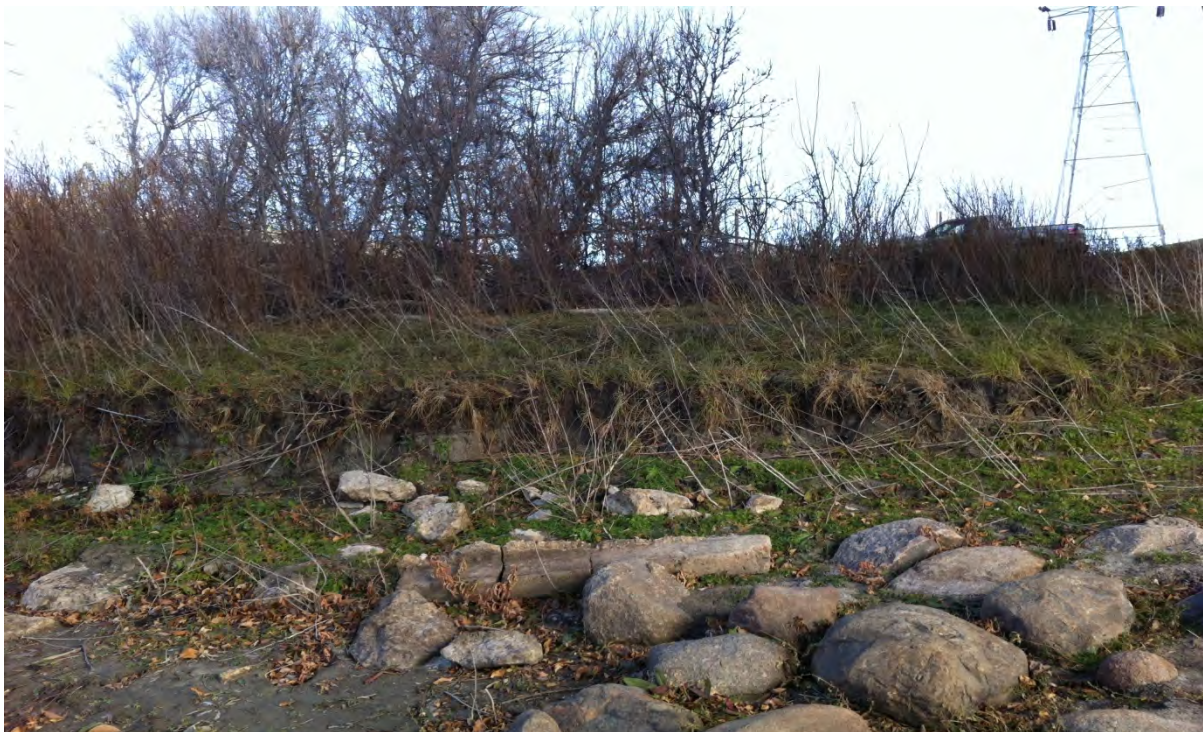
Photo 2: Erosion of riverbank toe, facing east.
