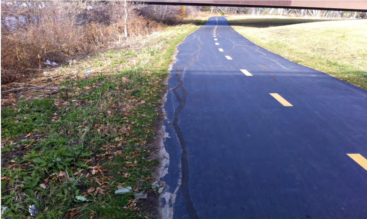
Photo 1: Cracking along the existing asphalt access road, mid-slope facing north.
