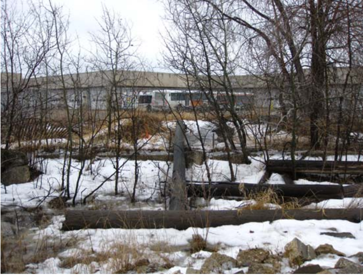
Looking east at area to be excavated. Note proximity of existing retaining wall. 2008-03-23_Field Excavation_P001
