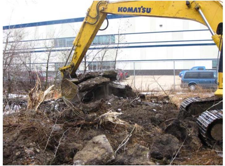
Looking north at excavated area. Note concrete slabs approximately 200 mm thick. 2008-03-23_Field Excavation_P006
