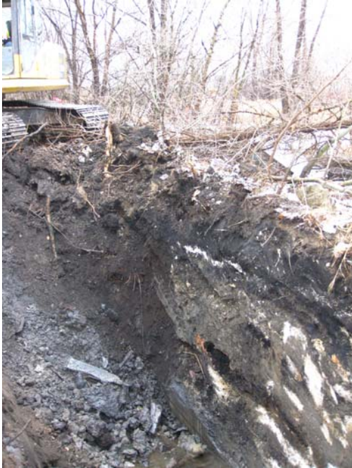
Looking south at excavated area (2 m wide x 4 m long x 3 m deep) adjacent existing retaining wall. 2008-03-23_Field Excavation_P013
