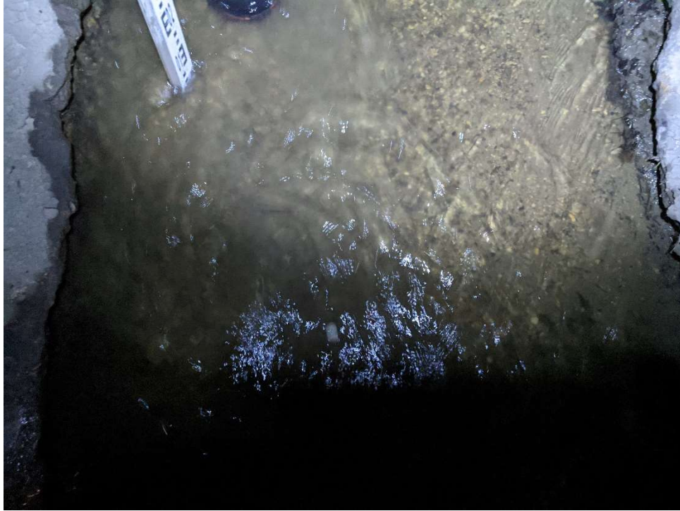
Photo Date: December 4, 2020 / at bend, looking down at invert (approx. 6:00 clock positioning)
