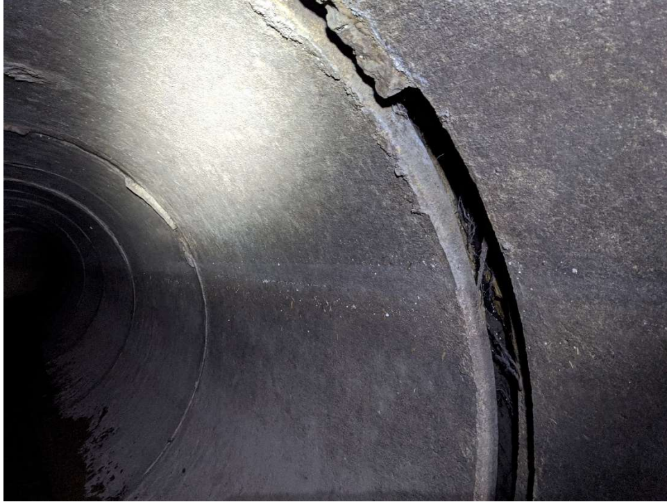
Photo Date: December 4, 2020 / Sta 1+46.5 (+/-) looking upstream at open joint
