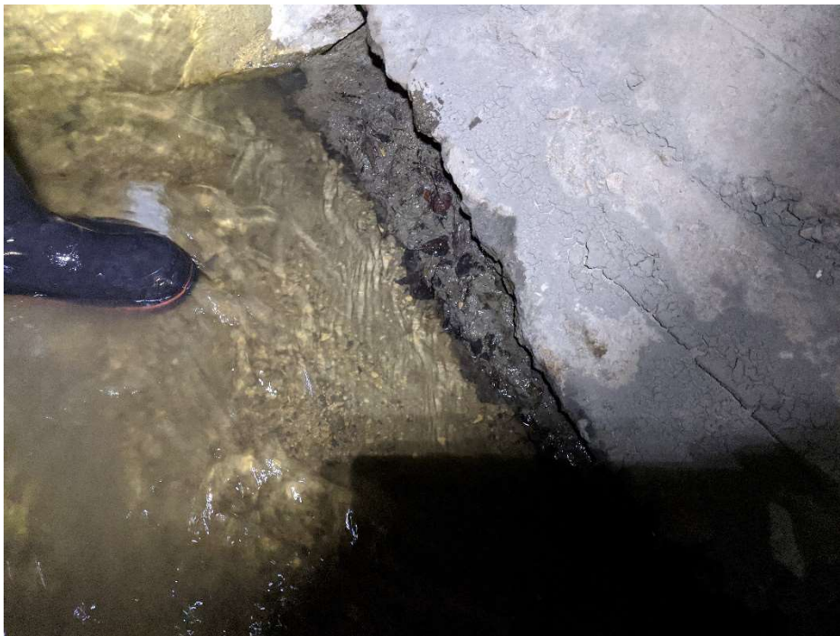
Photo Date: December 4, 2020 / at bend looking down at invert (5:30 approx. clock positioning)
