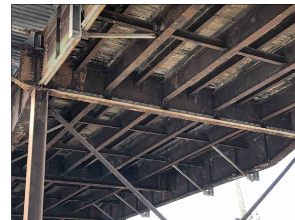
EXISTING CONDITION OF DIAPHRAGM BEAM ABOVE JARVIS AVENUE
