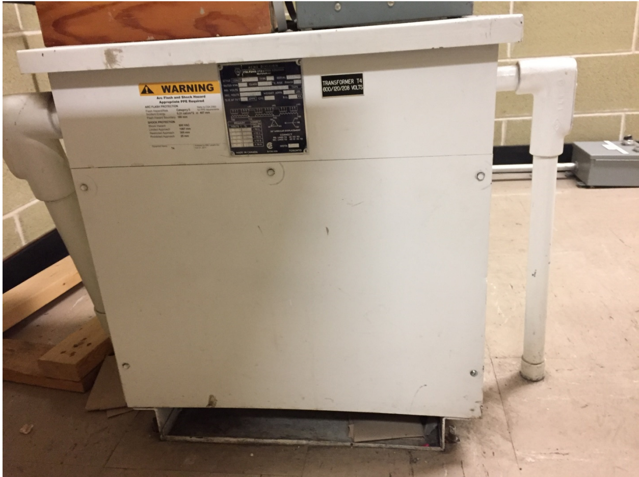
PHOTOGRAPH 5: McPhillips Regional Pumping Station - Electrical Room – facing east showing existing transformer T4.
