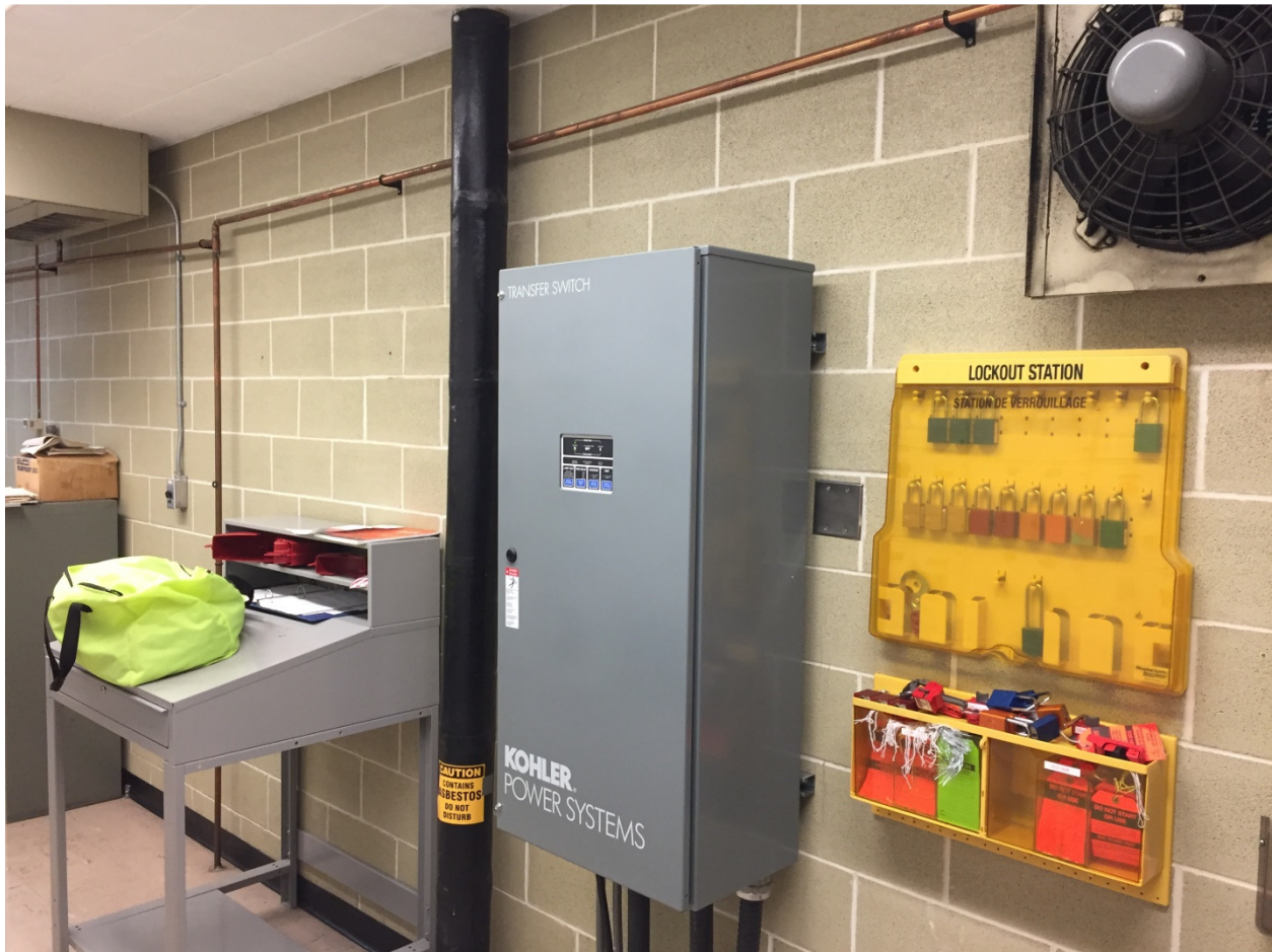
PHOTOGRAPH 1: McPhillips Regional Pumping Station - Electrical Room – facing southwest towards rainwater leader and copper piping to be relocated and existing automatic transfer switch (AST-M2E) to remain.
