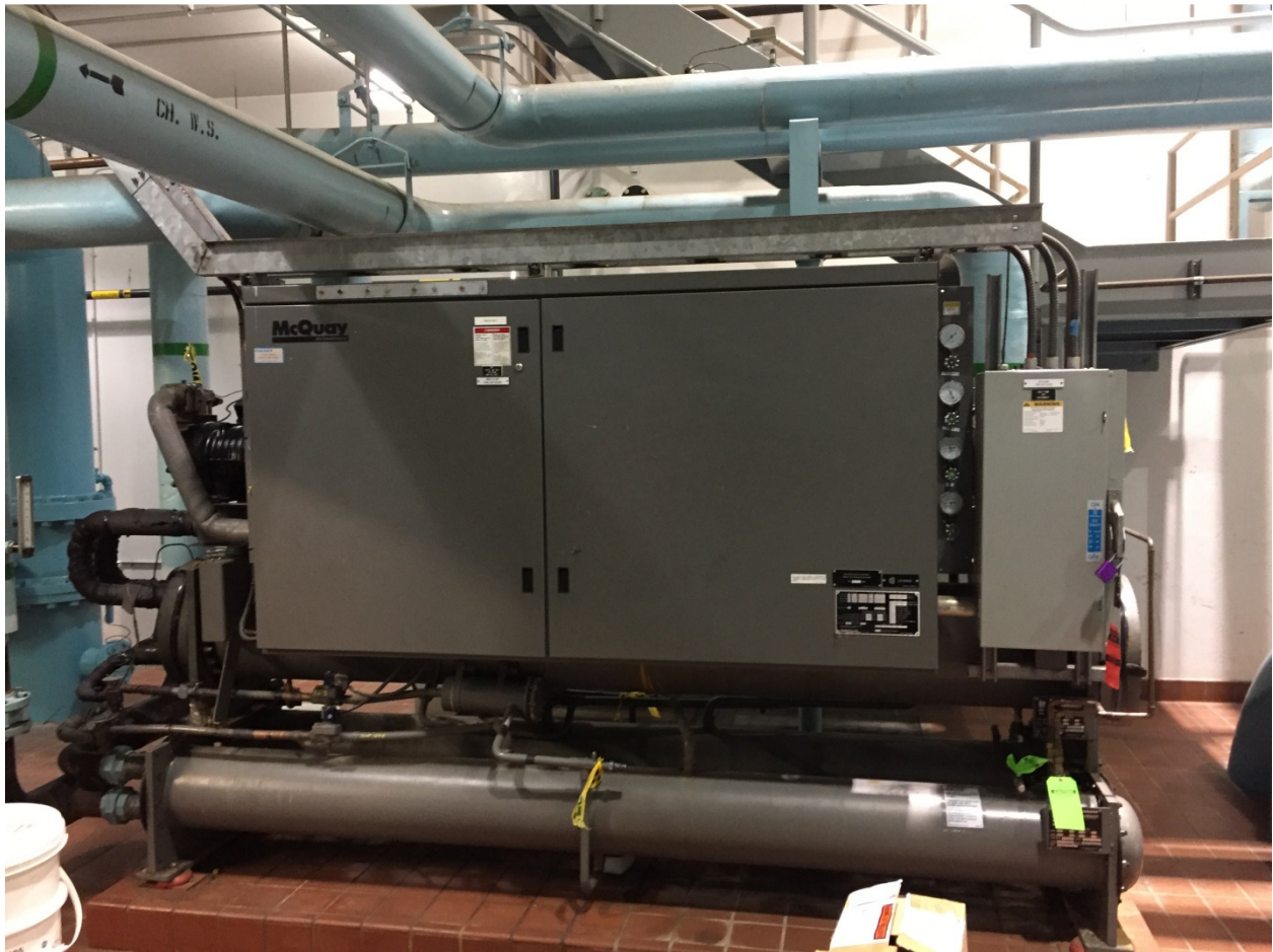
PHOTOGRAPH 10: McPhillips Regional Pumping Station - Pump Area – facing west showing existing chiller and piping.
