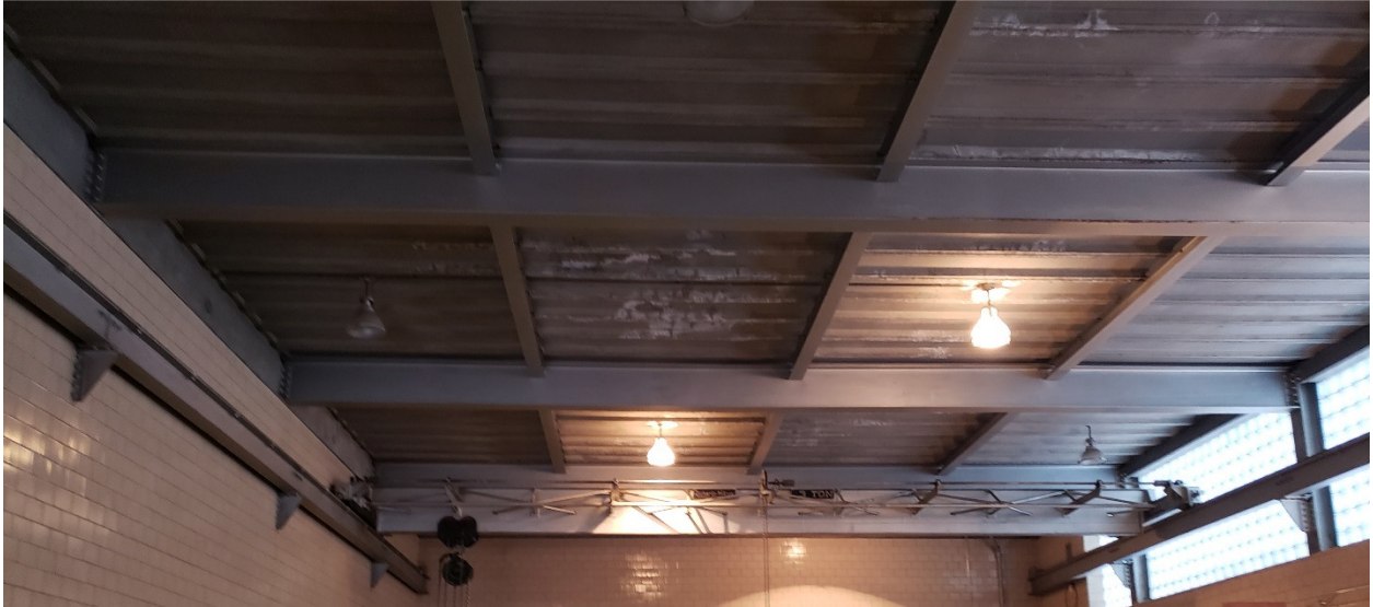
PHOTOGRAPH 36: Tache Booster Pumping Station – Main Level - facing northeast showing ceiling.
