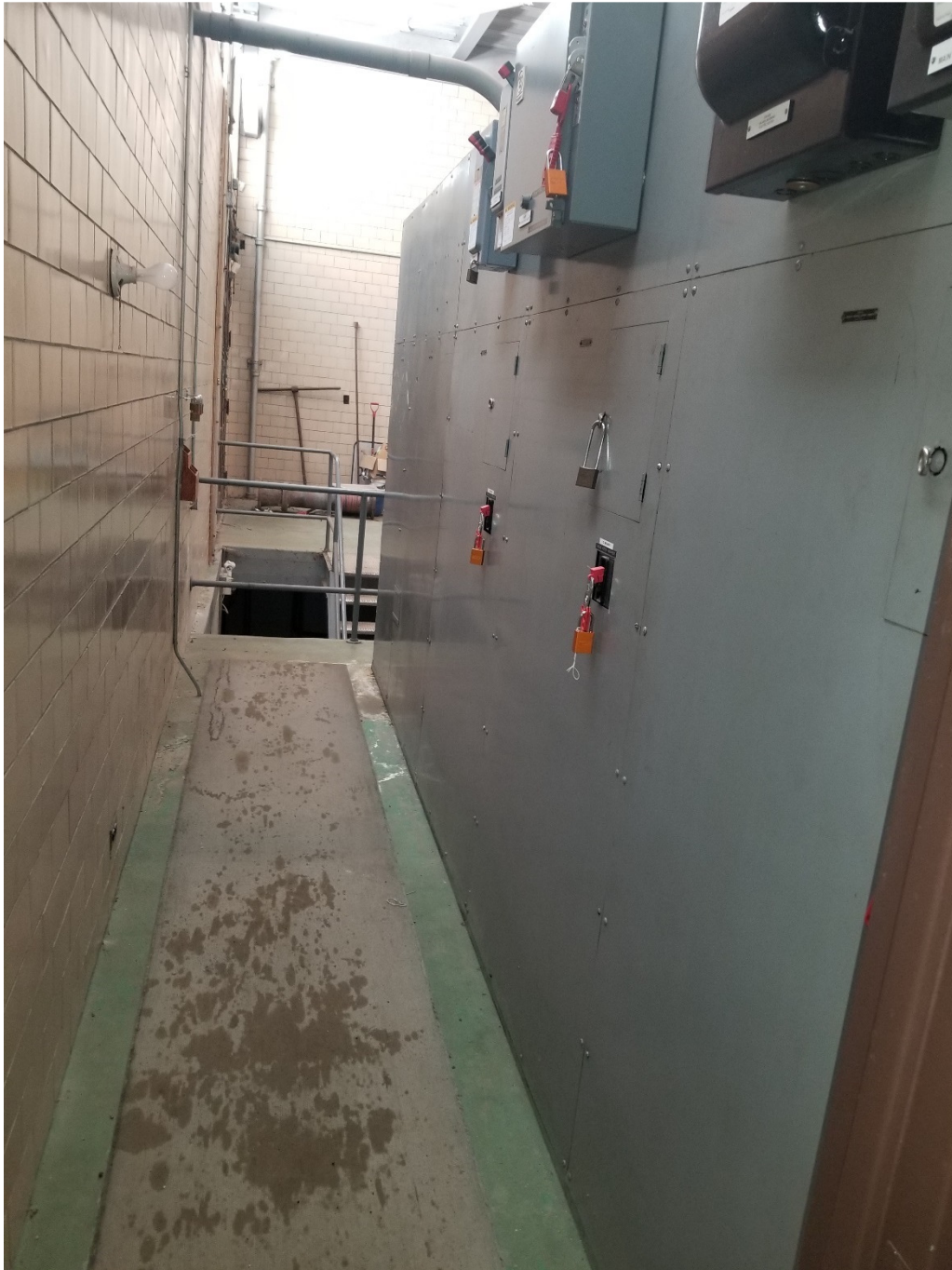
PHOTOGRAPH 34: Tache Booster Pumping Station – Main Level - facing southwest showing rear view of existing main 600V switchgear.
