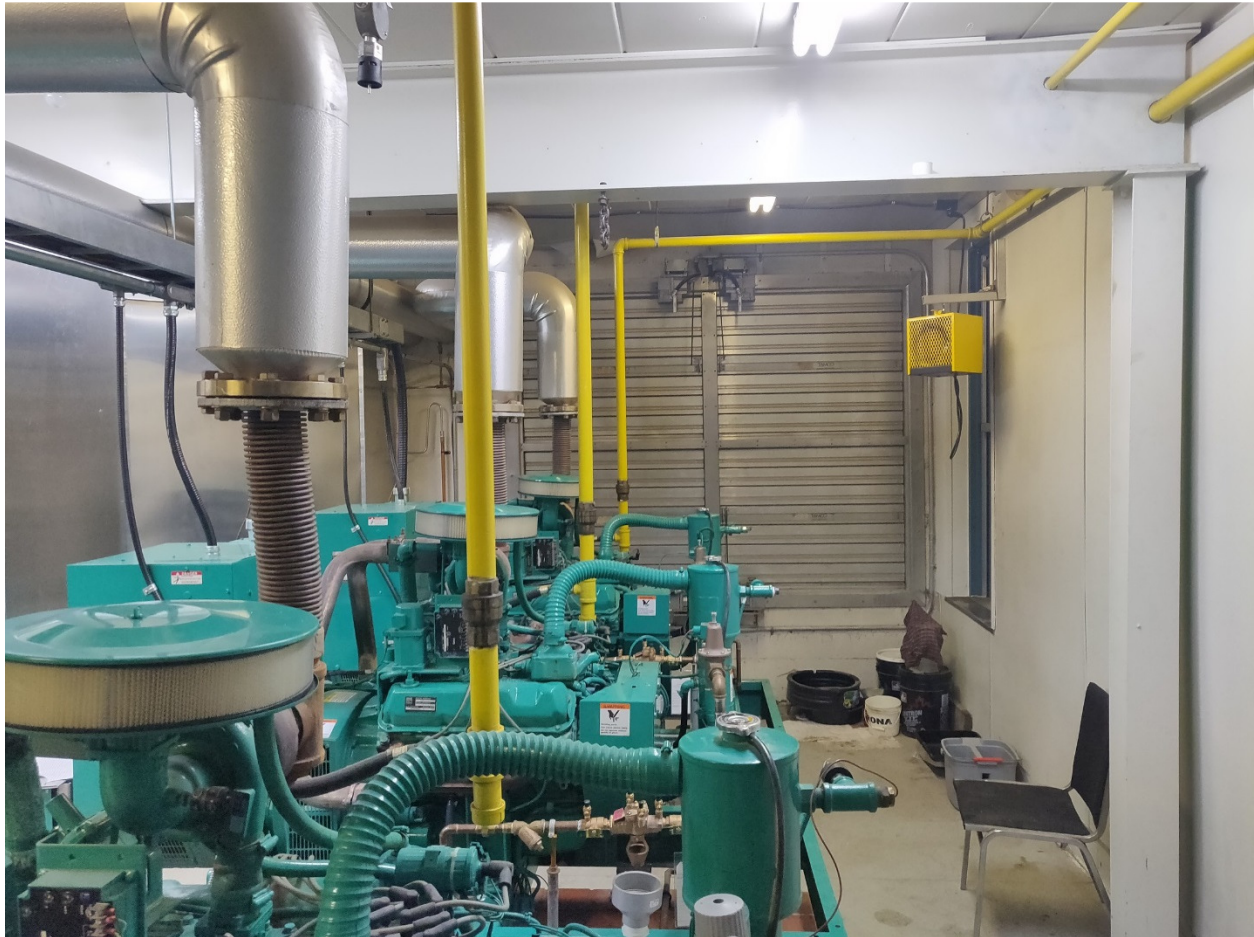
PHOTOGRAPH 26: McPhillips Regional Pumping Station – Collections Building – facing west showing Generator Room.
