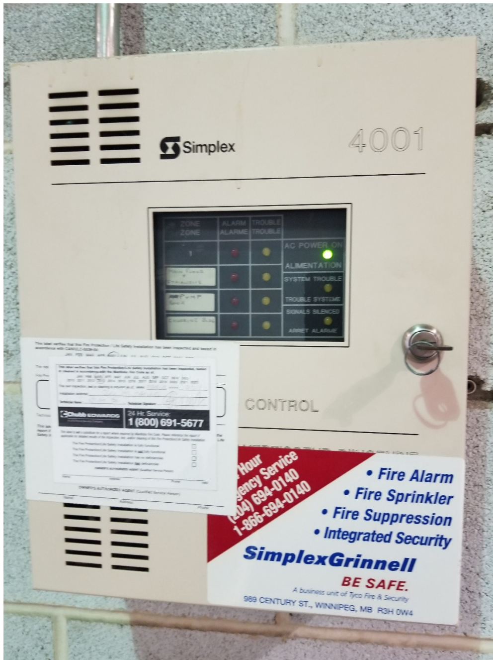
PHOTOGRAPH 15: Existing Fire Alarm Panel used in both McPhillips Regional Pumping Station and Tache Booster Pumping Station.
