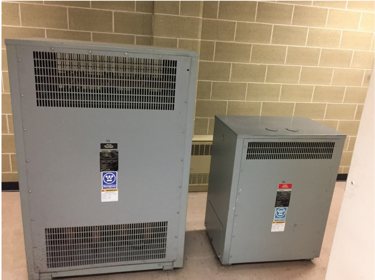
PHOTOGRAPH 4: McPhillips Regional Pumping Station - Electrical Room – facing east showing existing transformers T1 and T2.
