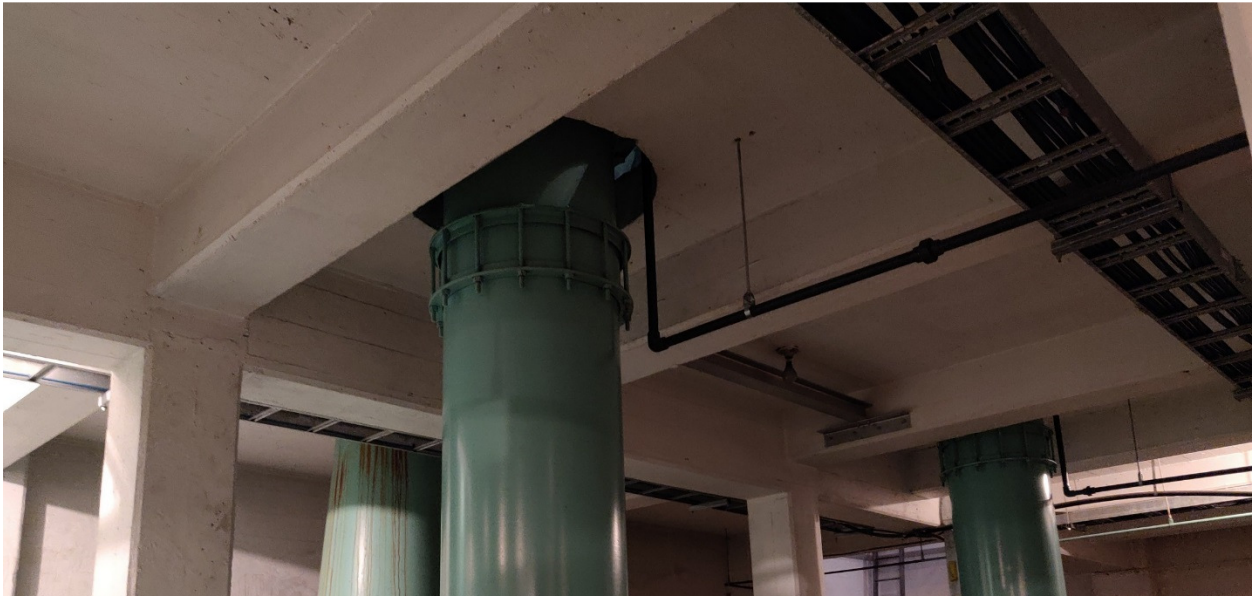
PHOTOGRAPH 39: Tache Booster Pumping Station – Lower Level – facing northeast showing ceiling.
