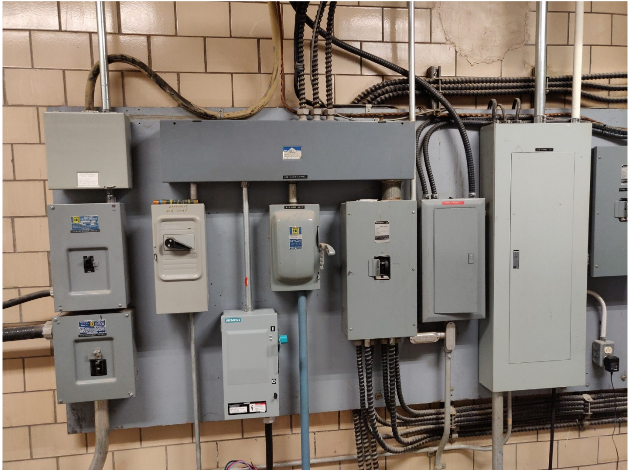
PHOTOGRAPH 28: McPhillips Regional Pumping Station – Collections Building – facing west in Electrical Room.
