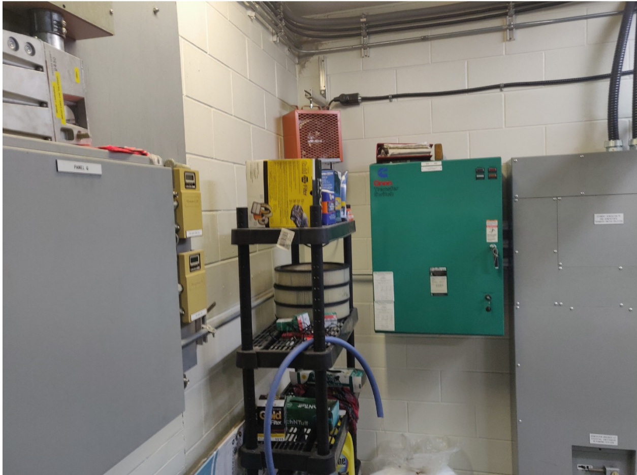
PHOTOGRAPH 24: McPhillips Regional Pumping Station – Collections Building – facing south in Generator Room.
