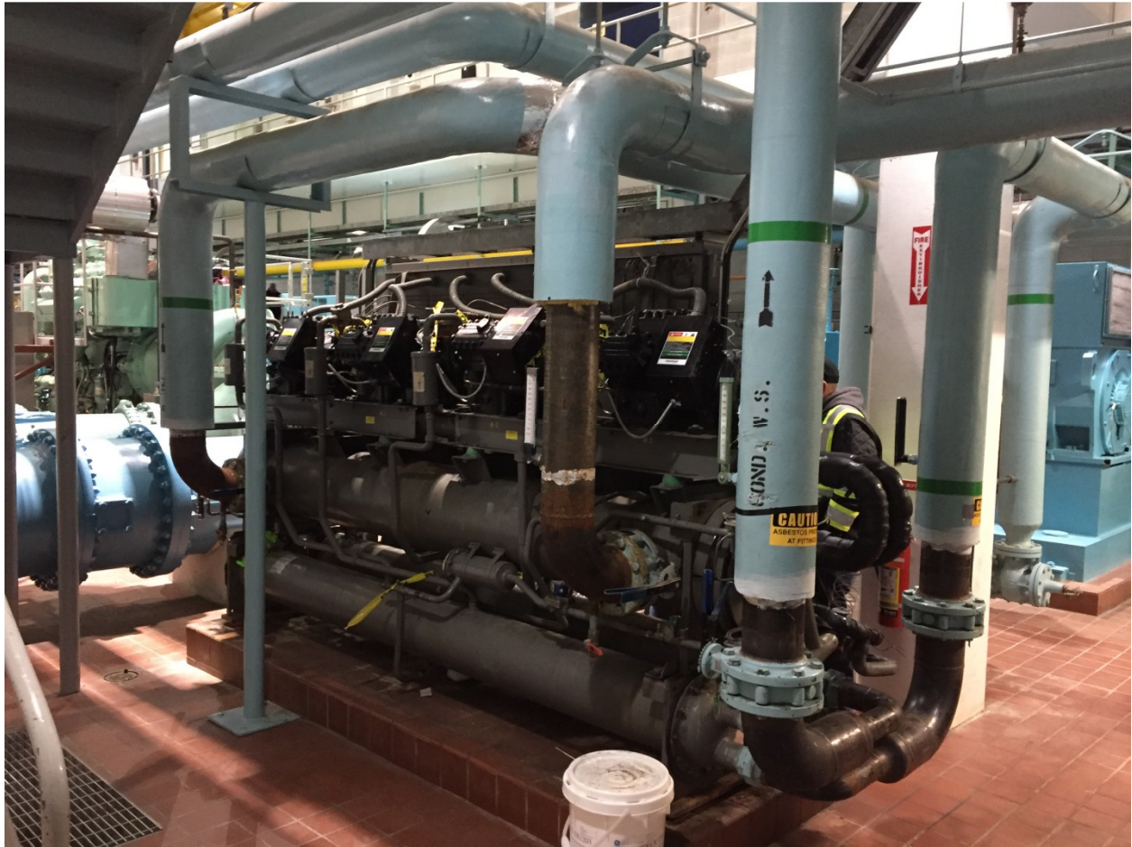
PHOTOGRAPH 8: McPhillips Regional Pumping Station - Pump Area – facing northeast showing existing chiller and piping.
