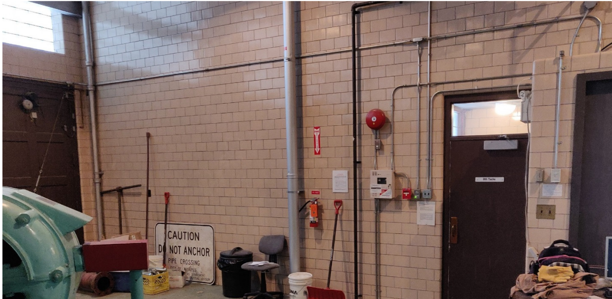
PHOTOGRAPH 37: Tache Booster Pumping Station – Main Level - facing southwest showing main entrance door.
