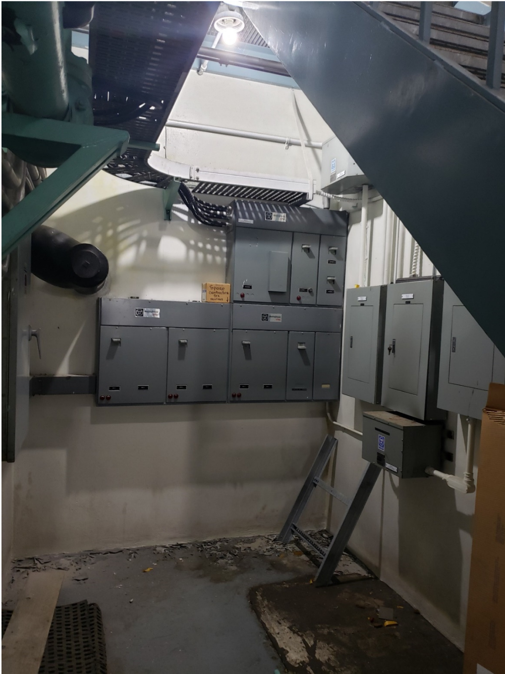
PHOTOGRAPH 22: McPhillips Regional Pumping Station - Chlorine Building Electrical Area –facing west showing existing equipment.
