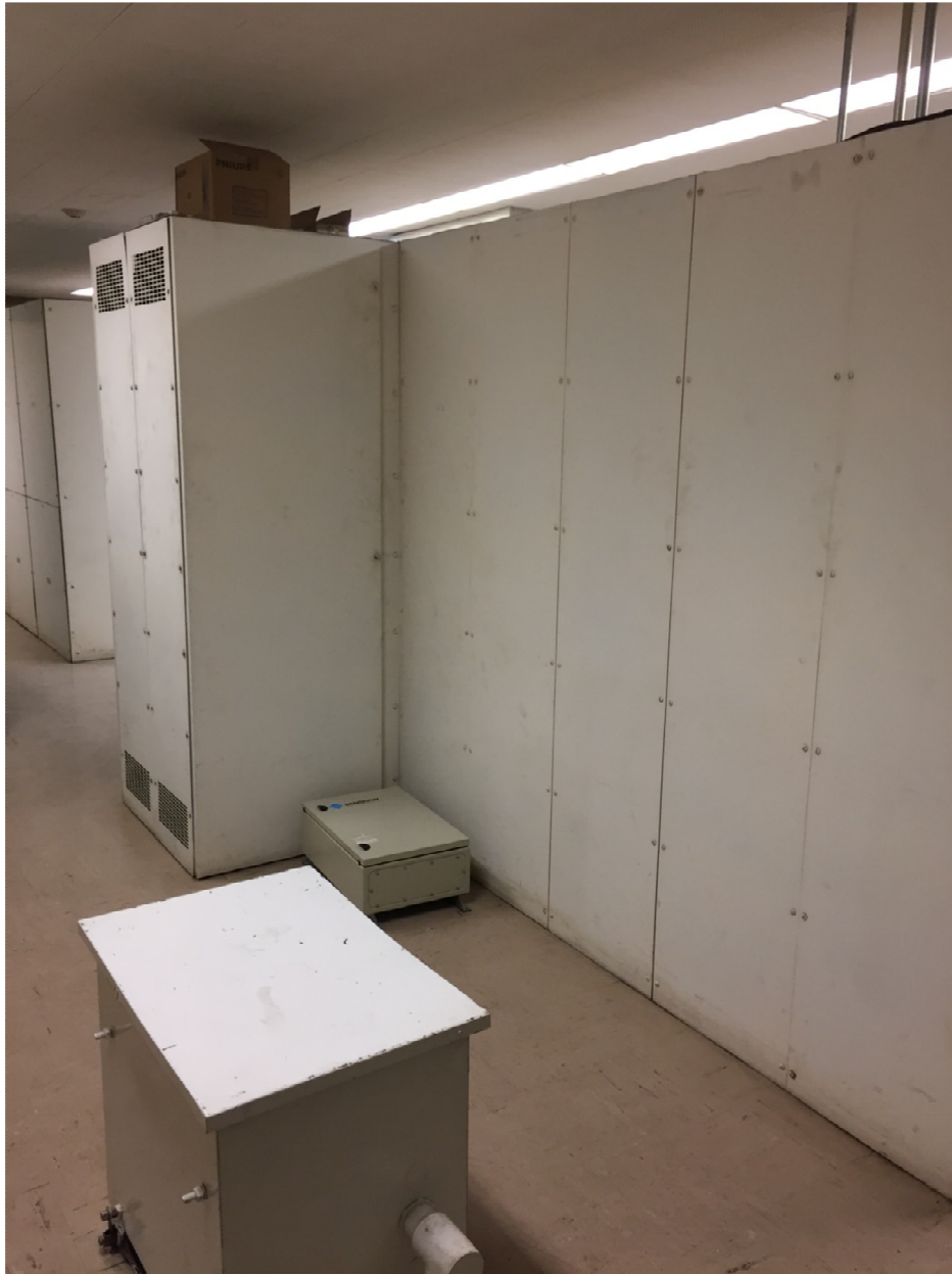
PHOTOGRAPH 3: McPhillips Regional Pumping Station - Electrical Room – facing south-southwest showing existing transformer T3 in the foreground and rear of existing 600V MCC and switchgear in background.
