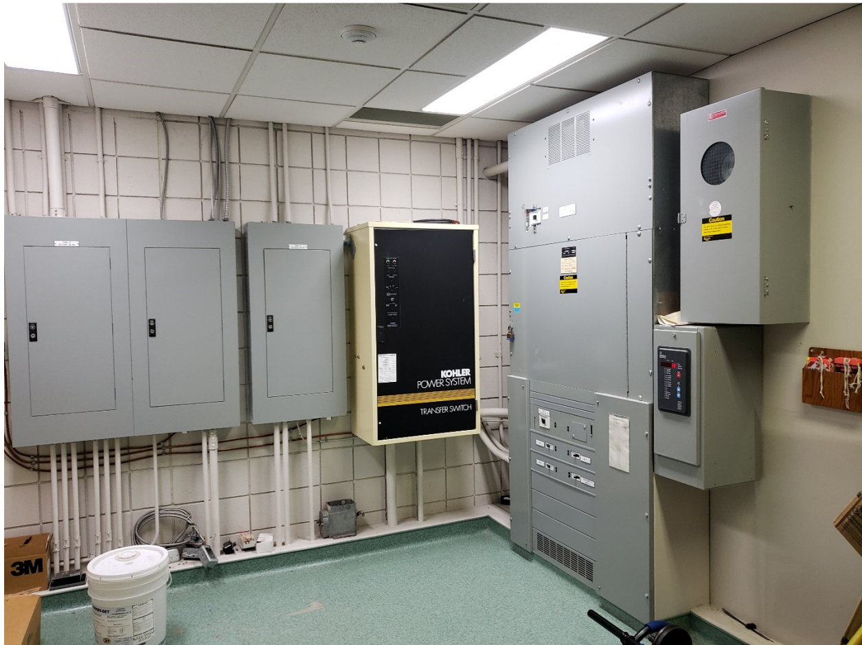
PHOTOGRAPH 27: McPhillips Regional Pumping Station – Control Centre – facing west showing Electrical Room.
