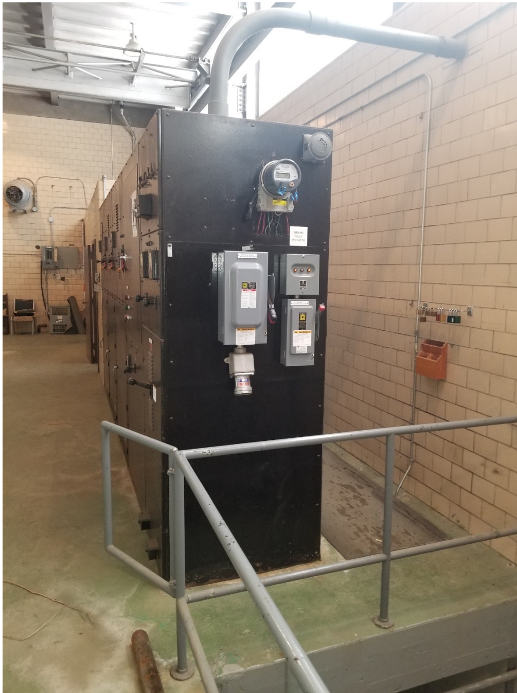
PHOTOGRAPH 33: Tache Booster Pumping Station – Main Level - facing east showing side view of existing main 600V switchgear.
