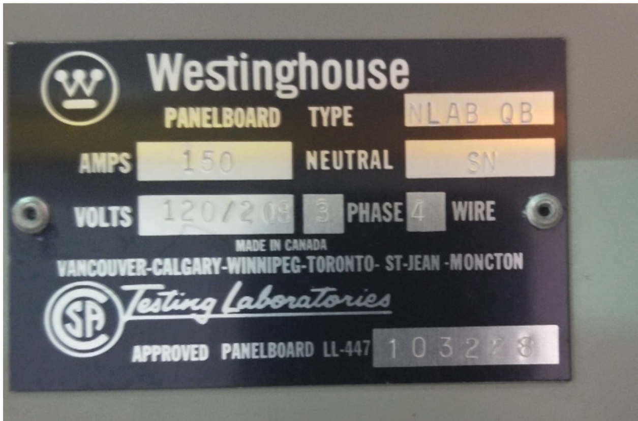
PHOTOGRAPH 16: McPhillips Regional Pumping Station - Part number for existing McPhillips Regional Pumping Station Panels LP-A and LP-B. LP-A is a 42 circuit version and LP-B is a 30 circuit version.
