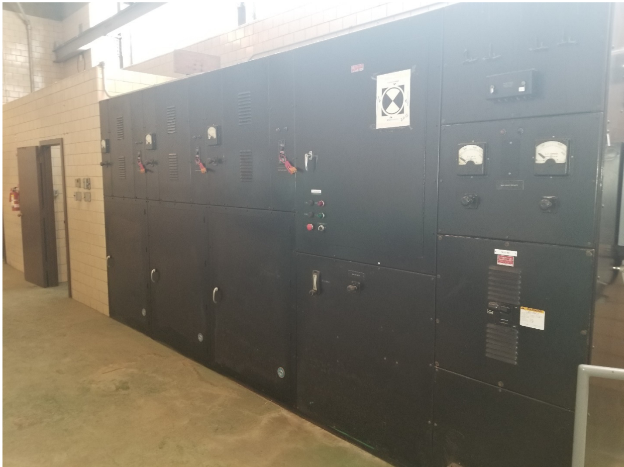
PHOTOGRAPH 32: Tache Booster Pumping Station – Main Level - facing east-southeast showing front view of existing main 600V Switchgear.
