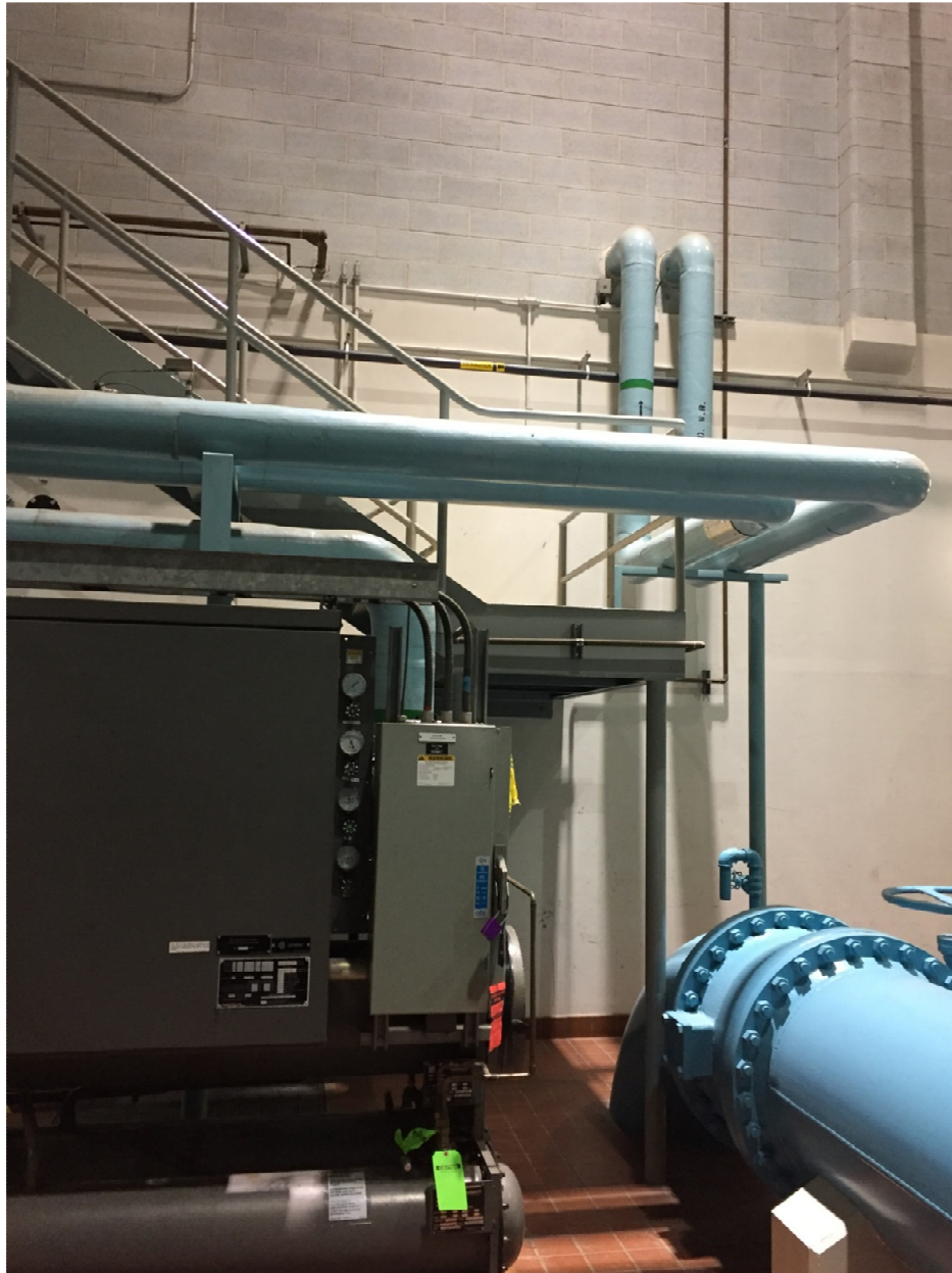
PHOTOGRAPH 9: McPhillips Regional Pumping Station - Pump Area – facing west showing existing chiller and piping.
