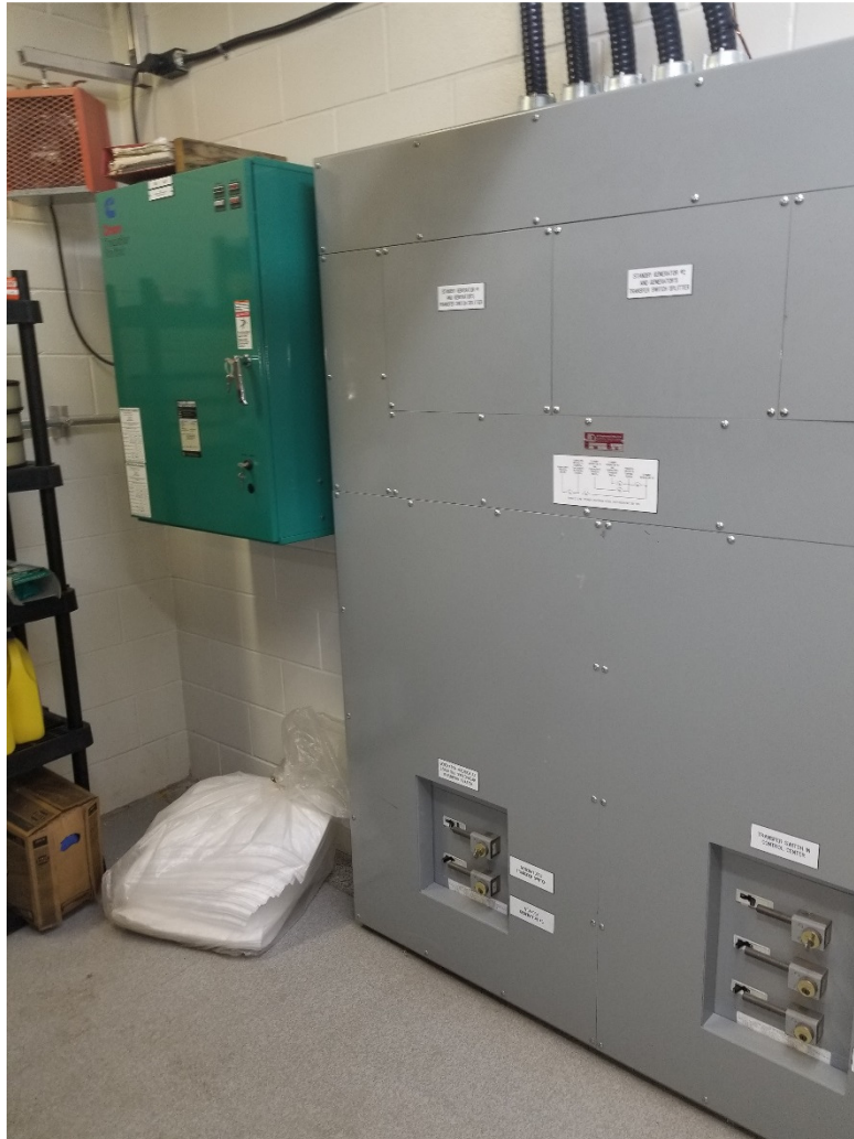
PHOTOGRAPH 25: McPhillips Regional Pumping Station – Collections Building – facing southeast in Generator Room showing existing switchboard SWBD-G1.
