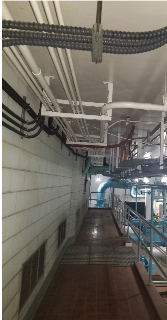
PHOTOGRAPH 14: McPhillips Regional Pumping Station - Pump Area – facing south showing walkway underneath mezzanine area.
