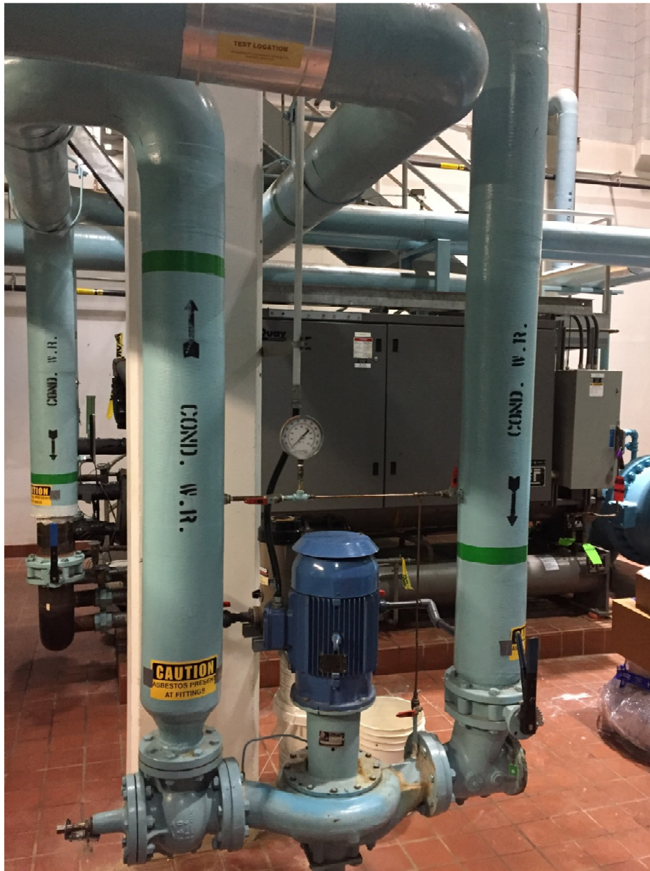
PHOTOGRAPH 11: McPhillips Regional Pumping Station - Pump Area – facing west showing existing pump, chiller and piping.
