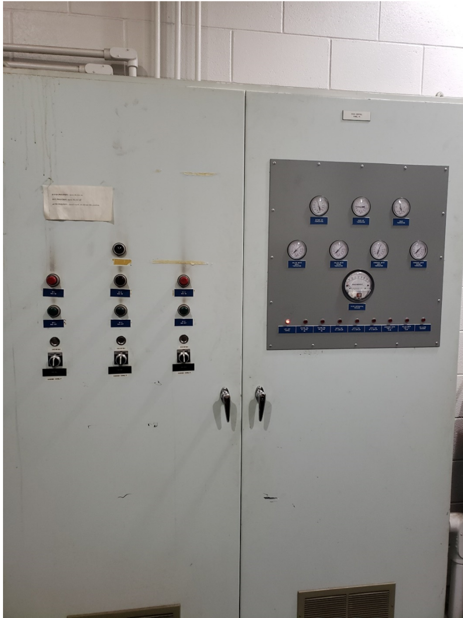
PHOTOGRAPH 19: McPhillips Regional Pumping Station –Mechanical Room – Facing east showing existing HVAC control panel.
