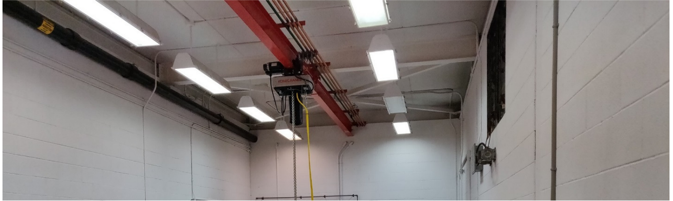
PHOTOGRAPH 23: McPhillips Regional Pumping Station – Chlorine Building - facing east showing ceiling in Chlorine Building Tank Room
