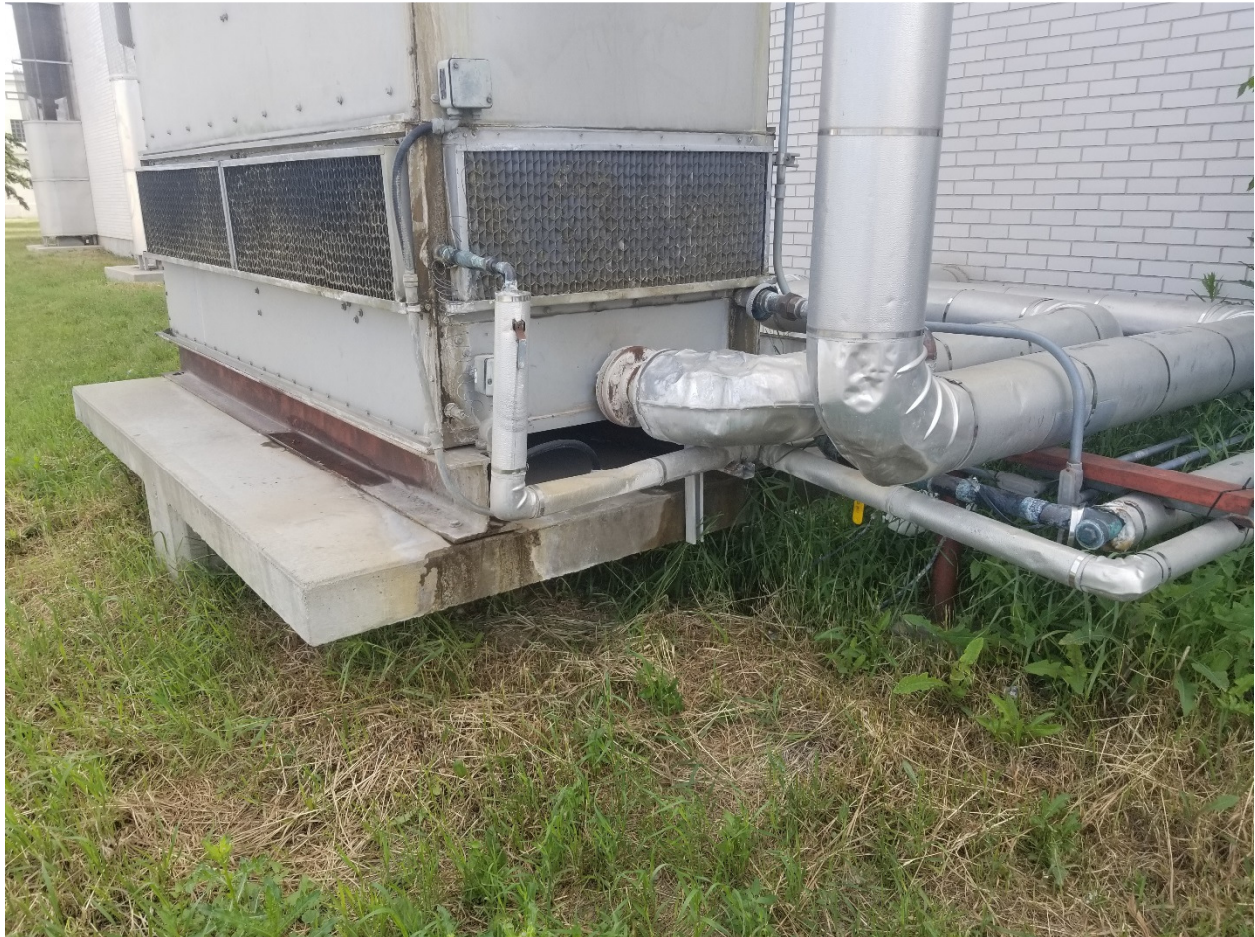
PHOTOGRAPH 31: McPhillips Regional Pumping Station – facing northeast showing existing cooling tower located on west side of main pumphouse building.
