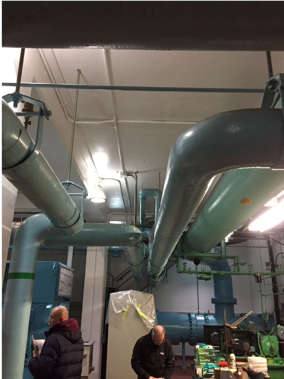
PHOTOGRAPH 12: McPhillips Regional Pumping Station - Pump Area – facing east showing existing piping.
