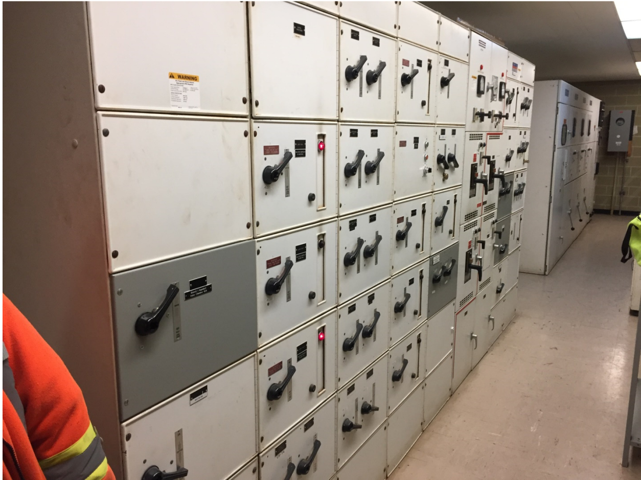
PHOTOGRAPH 2: McPhillips Regional Pumping Station - Electrical Room – facing south southeast showing existing 600V MCC and switchgear in foreground and existing 4160V switchgear in background.
