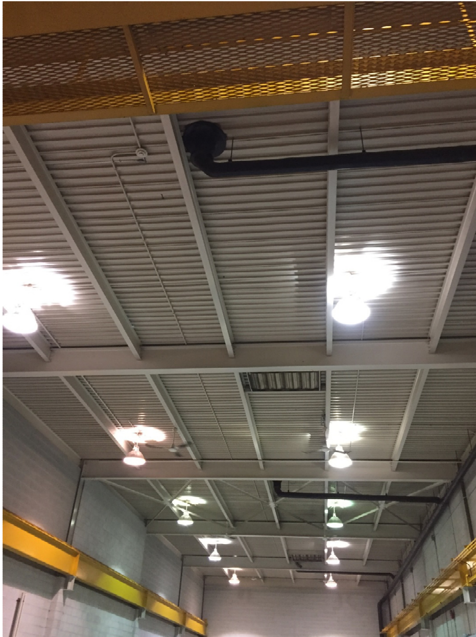
PHOTOGRAPH 7: McPhillips Regional Pumping Station - Pump Area – facing north showing existing high bay lighting.
