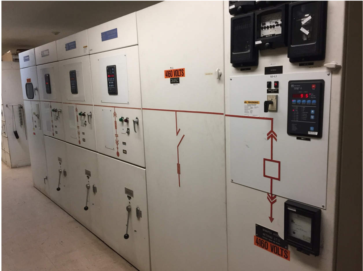
PHOTOGRAPH 6: McPhillips Regional Pumping Station - Electrical Room – facing northeast showing existing 4160V switchgear.
