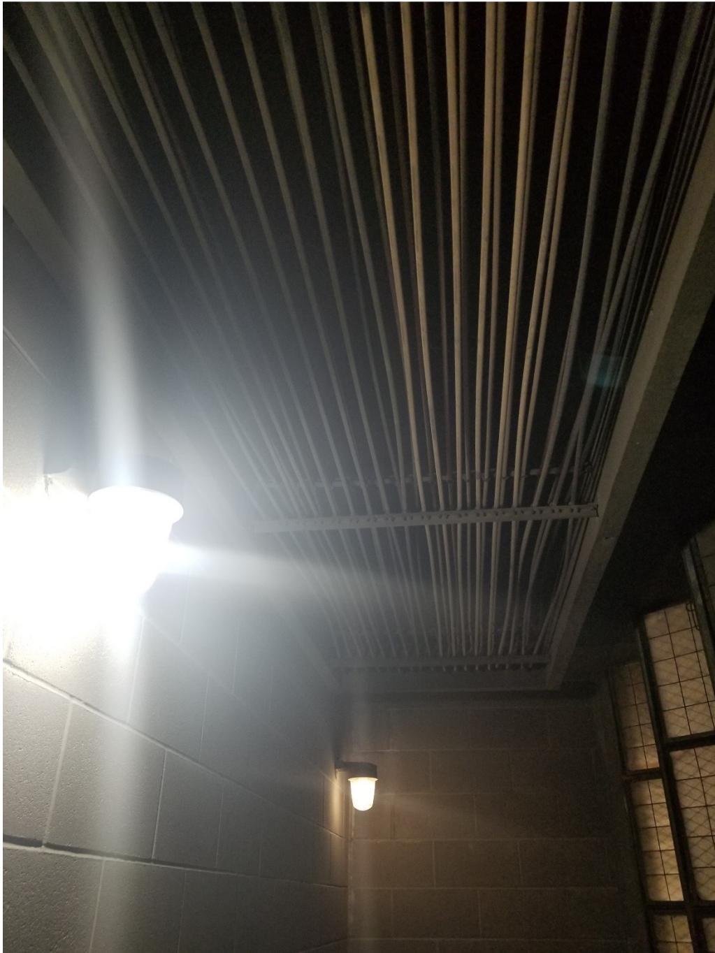
PHOTOGRAPH 21: McPhillips Regional Pumping Station – Electric Coil Room – showing location of new duct heater, HCE-M601.
