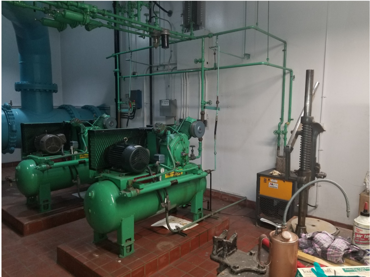
PHOTOGRAPH 13: McPhillips Regional Pumping Station - Pump Area – facing southeast showing existing air compressors.
