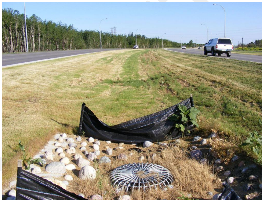
Figure 5.1 – Higher speed roadways with wide medians are to have appropriately sloped swales and standard ditch inlets.
