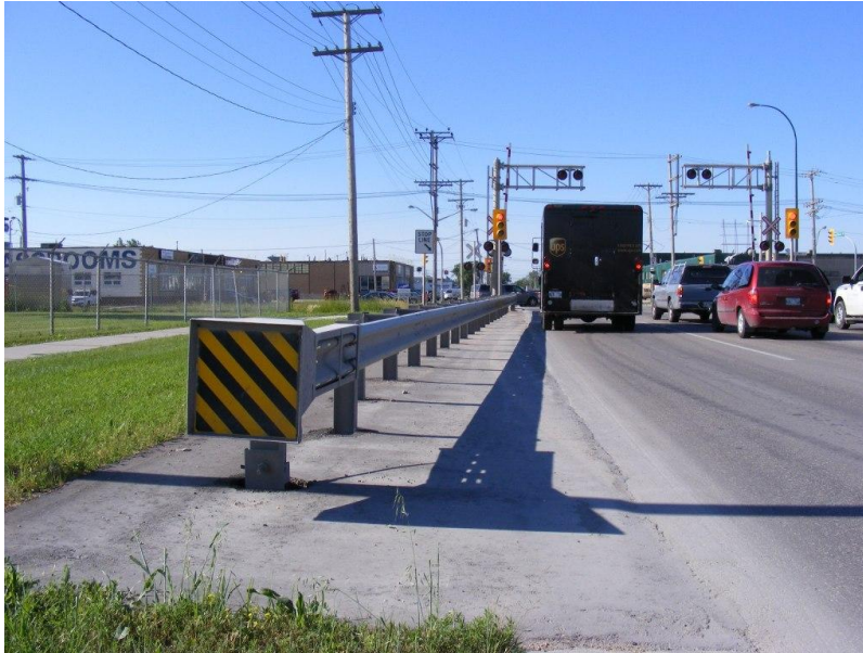
Figure 5.6 – W-beam guardrail installation on King Edwards demonstrates a flared end treatment and removal of curb for ease of snow clearing
