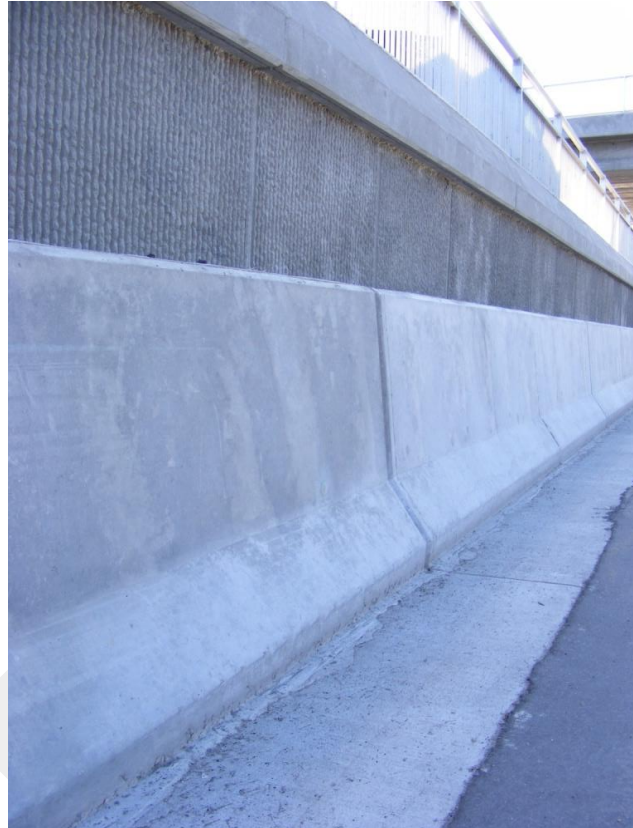
Figure 5.2 – Typical F-shape barrier in a TL-3 configuration due to the proximity of the retaining wall behind it
