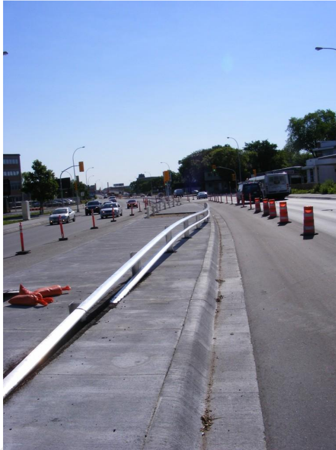
Figure 5.5 – Example of a new ABB installation on Disraeli Freeway that included a horizontally flared buried end.
