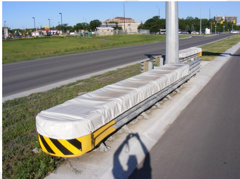
Figure 5.8 – Typical OHSS protection utilizing crash attenuators with an extension panel for low angle protection
