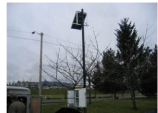
Pole mounted solar power system.
