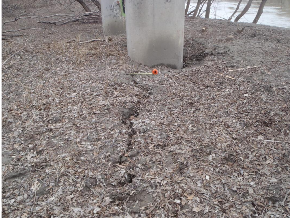
Photo 01: Tension Crack in the Vicinity of the South Pier (looking west).
