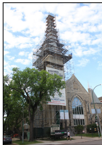
The successful reroofing of the spire at Augustine United Church, 444 River Avenue, 2021. (M. Peterson)
