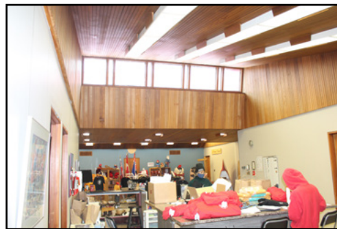
St. Boniface Health Unit Building, 233 Boulevard Provencher, ceiling, 2021. (M. Peterson)
