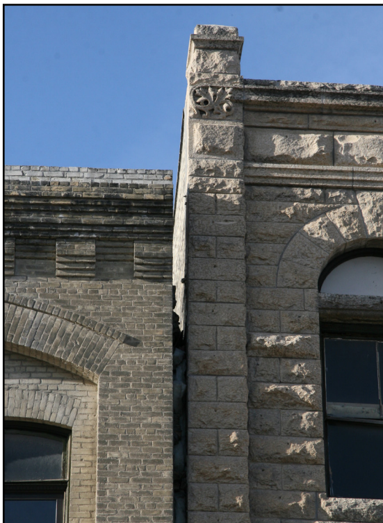
Thomas Scott Memorial Orange Hall, south wall pulled away from neighbouring building
