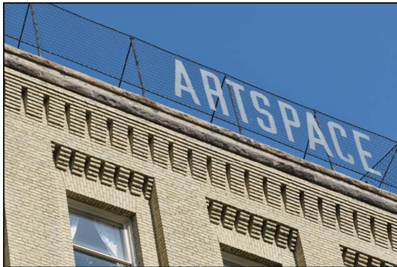
Roof sign fence, Gault Building, "Artspace", 100 Arthur Street, List of Historical Resources (G. Cline)
