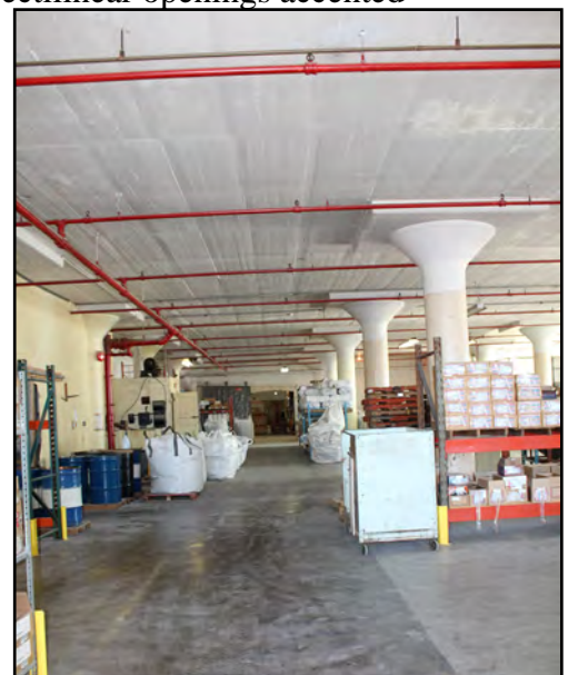
Second floor of the former track warehouse (west end of the structure)
