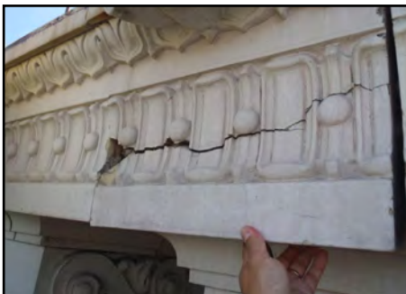
Close-up of cracked/fractured terra cotta on the cornice
