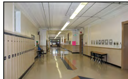
Wide, high ceilinged central hallways were a common feature of Winnipeg School division structures
