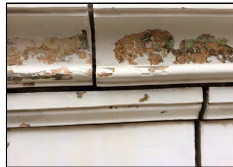
An example of the damage to the terra cotta, NWCTA Building
