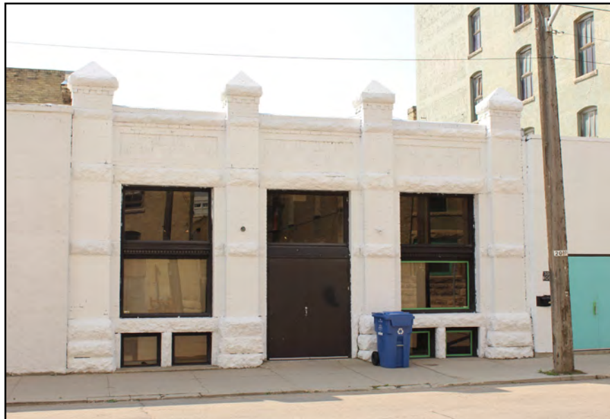
Toronto Hide and Wool Company Building, 200 Princess Street. The original brick exterior was painted.
