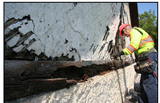
Workers removing rotting stucco and wood elements in preparation for new cladding
