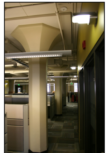
423 Main Street, Canadian Wheat Board Building, concrete columns on the seventh floor
