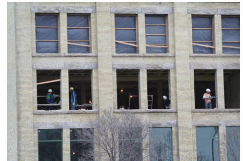
Renovation work continues on the front (south) façade windows of the Kemp Building, November 2011.
