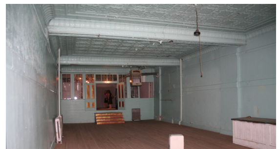
Ground floor space with mezzanine to the rear and ornamental tin ceiling
