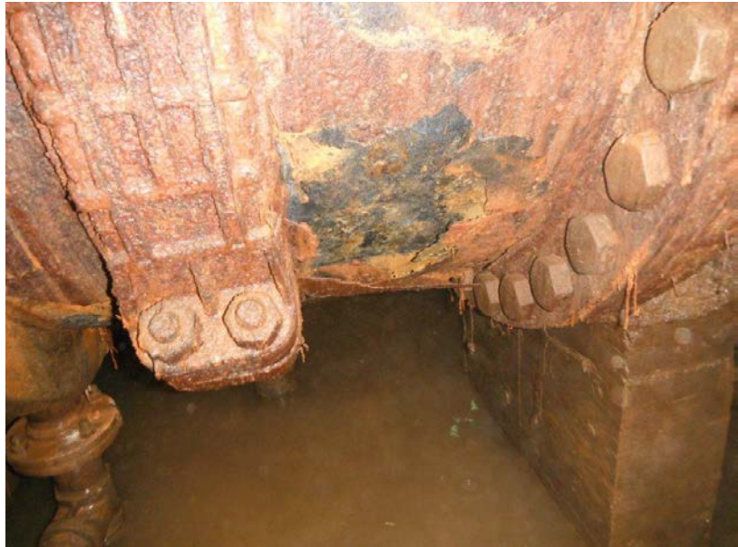
Figure 22: Fasteners, Condition Grade 2. Interconnecting Pipework Body Condition Grade 3
