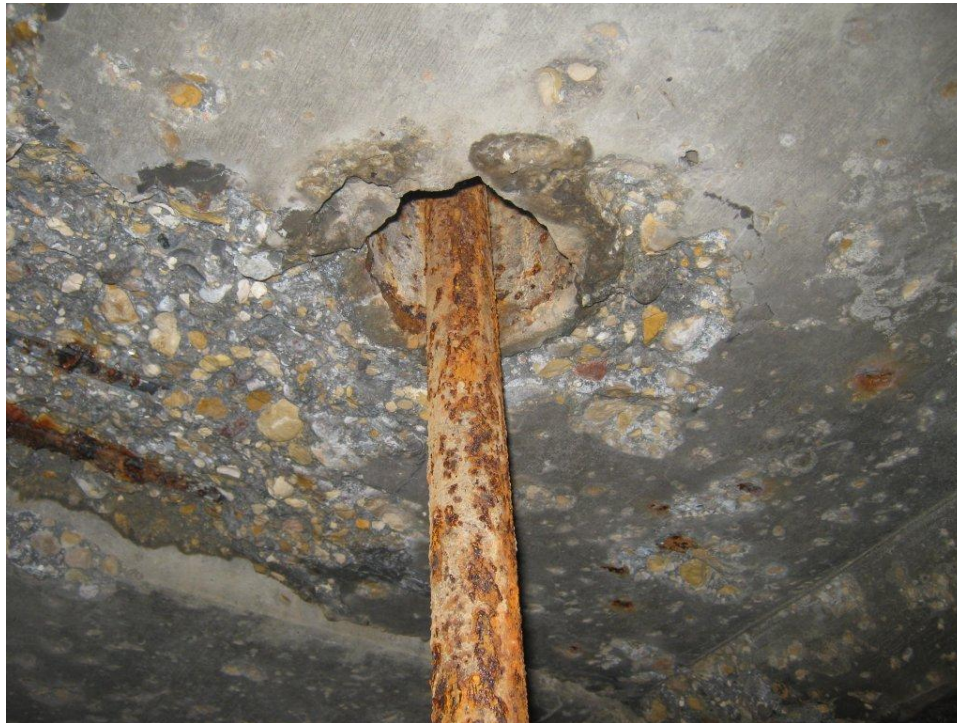
Figure 17: Example of Removable Roof Slab with Condition Rating of 4. Efflorescence and/or Water Infiltration
