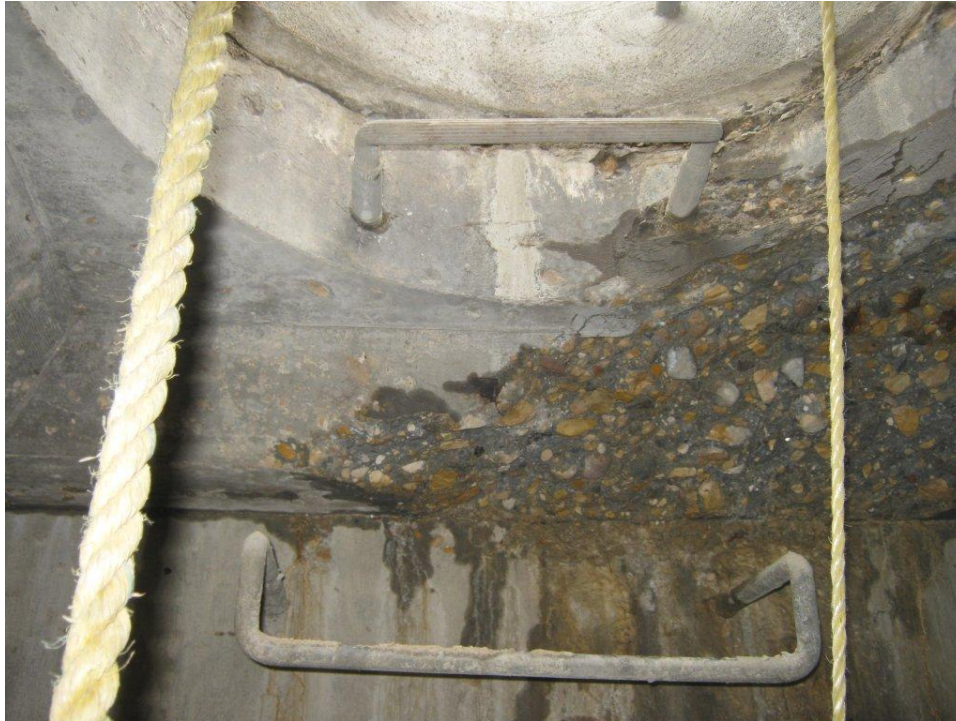
Figure 18: Example of Conditions for the Roof (4. Efflorescence and/or Water Infiltration) and Rungs (2. Normal Wear)
