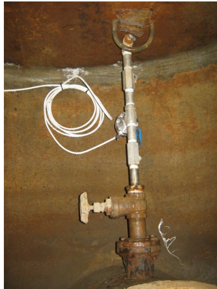
Figure 19: Example of Pressure Transmitter (QIB-599-PT) with Condition Rating 1. Good.
