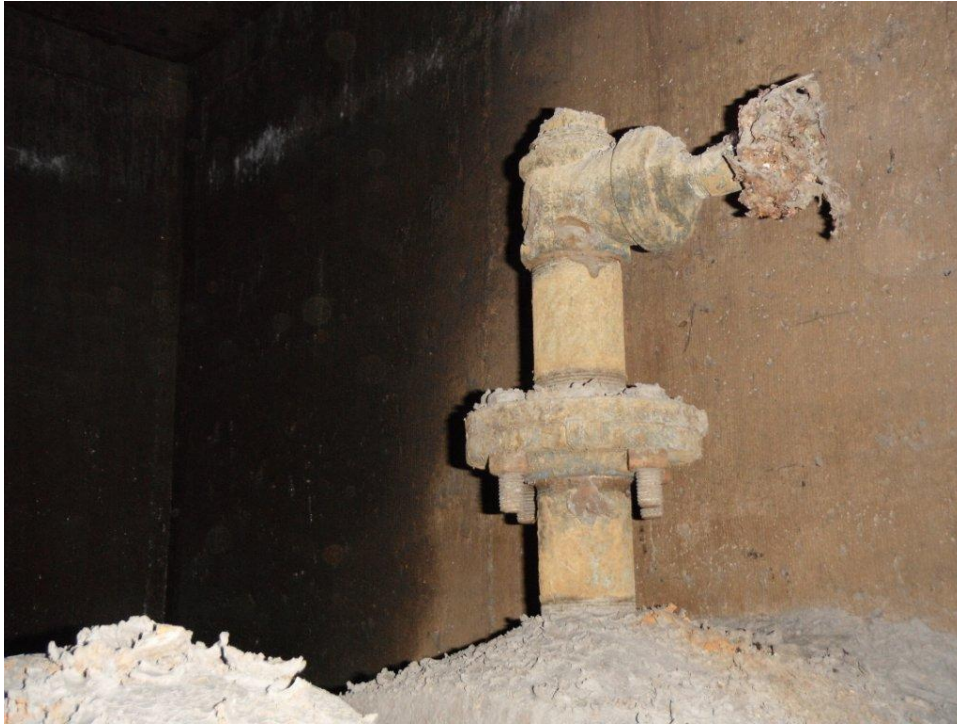
Figure 21: Example of Air Release Valve Body (2. Slight Missing Coating and Corrosion of Metal), Fastener (2. Slight Corrosion), and Port (3. Moderate Missing Coating and Corrosion of Metal)
