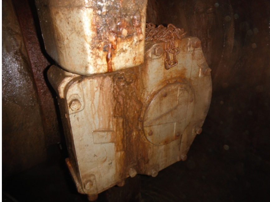
Figure 20: Example of Gearbox Condition with Rating of 2. Slight Missing Coating and Corrosion of Metal
