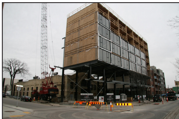
Construction continues on the residential tower to the east of the Pumping Station, 2019. (City of Winnipeg)
