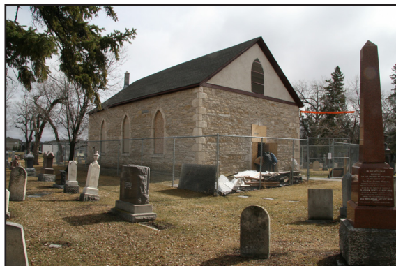
Completed south and west façades, Kildonan Presbyterian Church, John Black Avenue, 2020. (City of Winnipeg)
