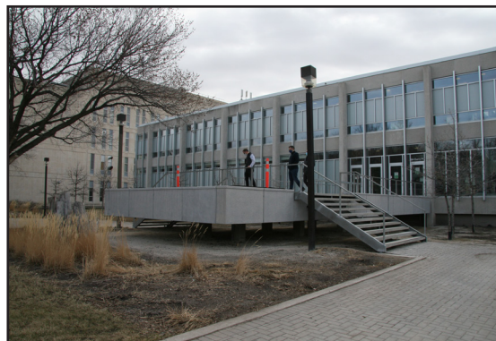
Work underway on the north façade entrance, J.A. Russell Building, 83 Dafoe Road, 2009. (City of Winnipeg)
