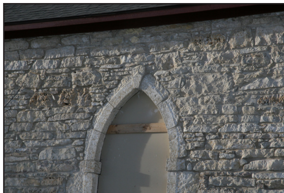
Completed restoration on window and wall, east façade, Kildonan Presbyterian Church, John Black Avenue, 2020. (City of Winnipeg)
