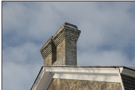
Archbishop's Residence, 151 avenue de la Cathédrale, south end brick chimney prior to repairs, 2020. (City of Winnipeg)
