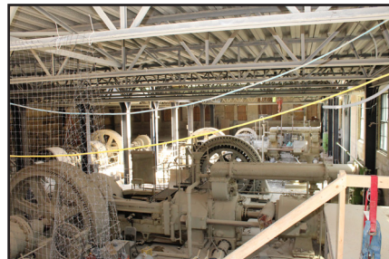
James Avenue Pumping Station, 109 James Avenue, view of basement pumping machinery and new flooring above, 2017. (City of Winnipeg)
