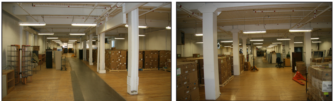
Ground floor of the Paulin-Chambers Building, 311 Ross Avenue, showing both steel (left) and timber (right) structural systems, 2018.
