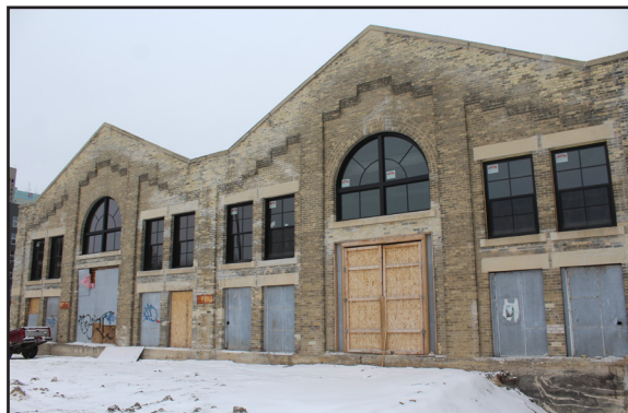
James Avenue Pumping Station, 109 James Avenue, east façade with newly installed window units, 2017. (City of Winnipeg)
