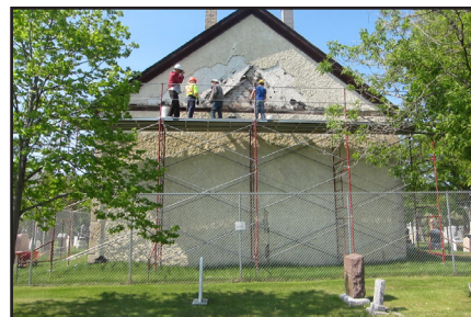
Work begins on stucco removal, north façade, Kildonan Presbyterian Church, John Black Avenue, 2015. (City of Winnipeg)
