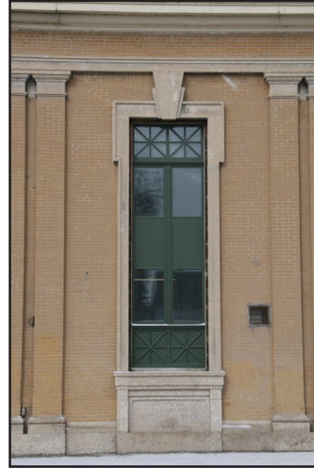
New window unit and ornamental detailing, east façade, Ukrainian Labour Temple, 591 Pritchard Avenue. (City of Winnipeg)
