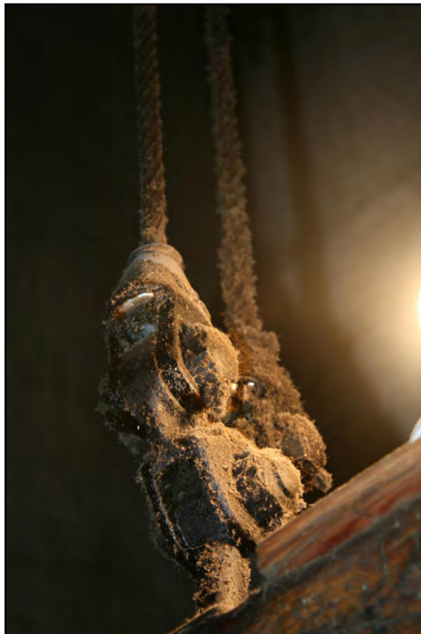
Original elevator equipment, G.F. and J. Galt Block
