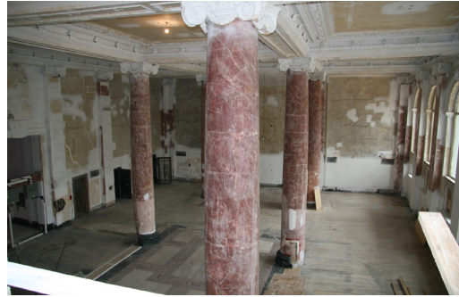
Banking Hall, 504 Main Street, after removing the mould from the interior finishes.
