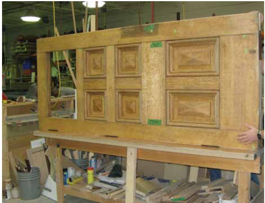
Preserving the wood doors of the Langevin Block in Ottawa included carefully dismantling the doors to permit the damaged and decayed wood to be repaired.
