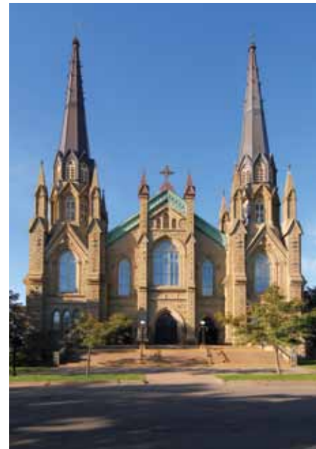
It is important to consider the expected life span of all elements that make up a roof assembly when repairing or replacing a roof such as this one on St. Dunstan's Basilica in Prince Edward Island. Roofing materials, such as copper and slate, need to be matched with flashings of a similar life span.
