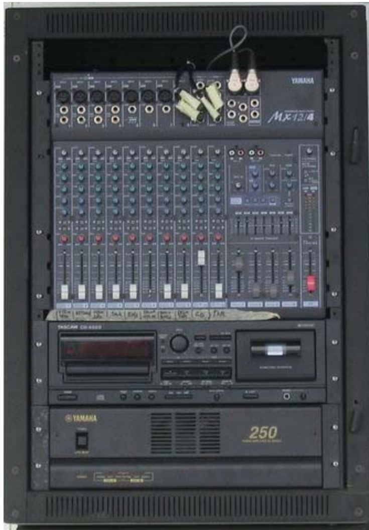
Sound System – Mixing Board
