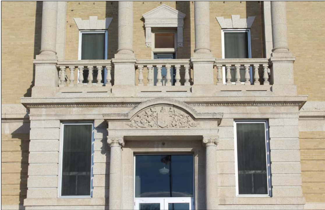
Plate 16 – Administration Building, Manitoba Agricultural College, 139 Tuxedo Avenue, detail of front (south) entrance, 2018. ( M. Peterson, 2018. )
