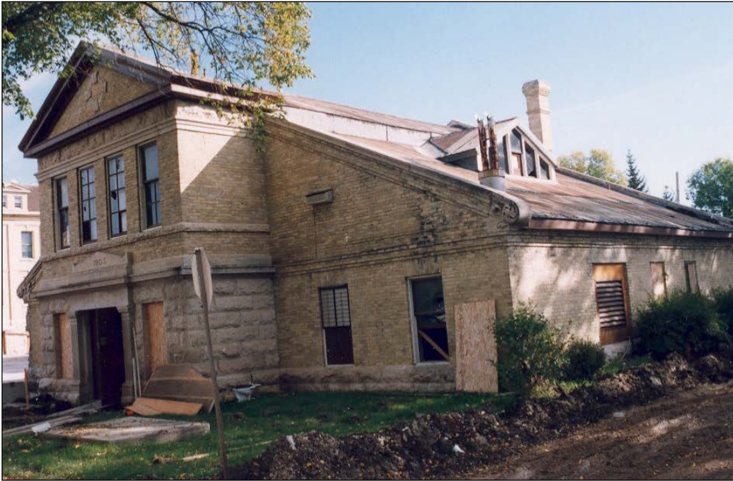
Plate 22 – Power House, Manitoba Agricultural College, 139 Tuxedo Avenue, front (west) and south façades, 1995. (M. Peterson, 1995.)
