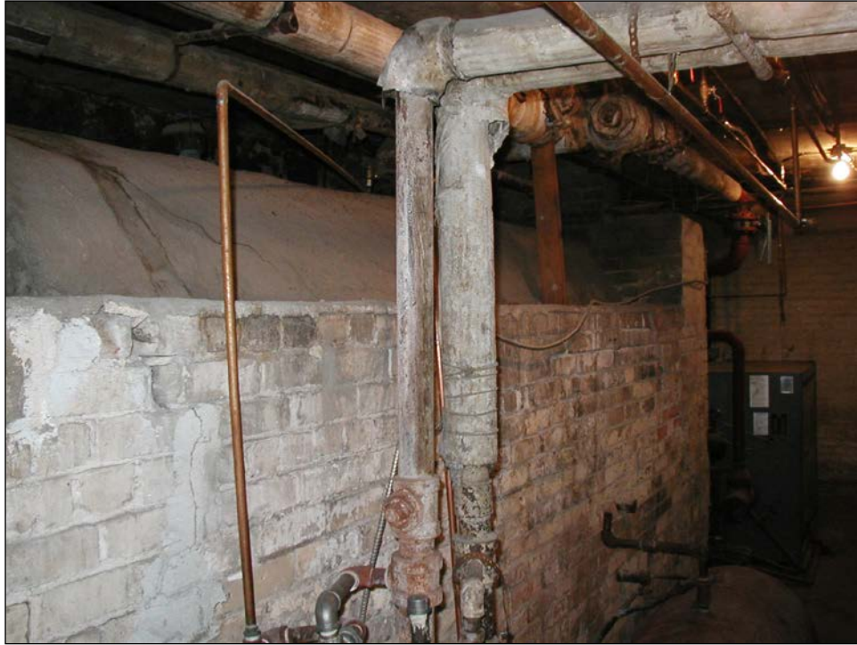
Plate 12 – Windsor Hotel, 187 Garry Street, basement boiler. (M. Peterson, 2005.)
