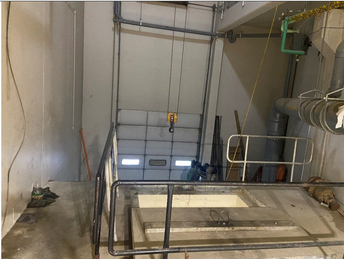
Exchanger Unload Location Inside
