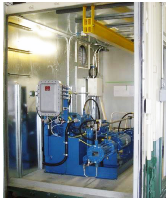
Construction of hydrogen station illustrating compressor room at one end of 12m container
