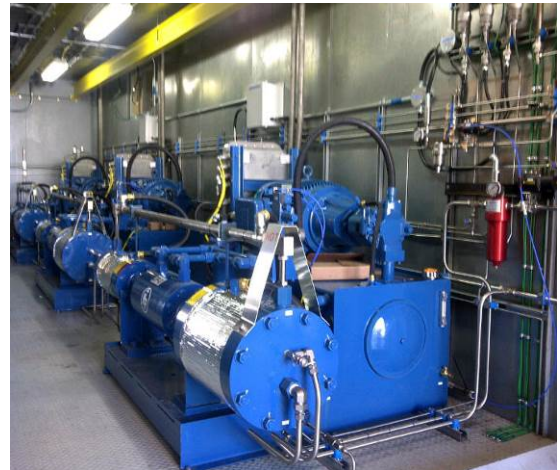
3 compressors in one 12 m container
