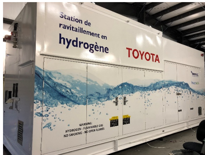
Figure 1. Powertech's Containerized 700 bar dispenser in Quebec City, Quebec.
