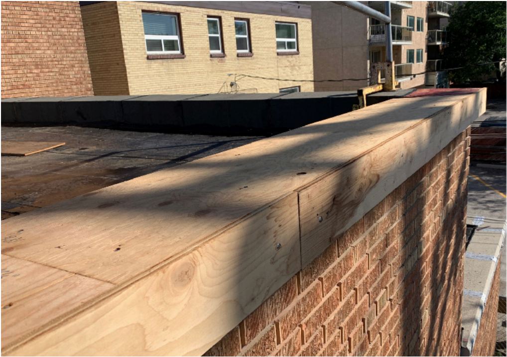
Plywood sheathing to be applied to all roof membrane and flashing mateable surfaces.
