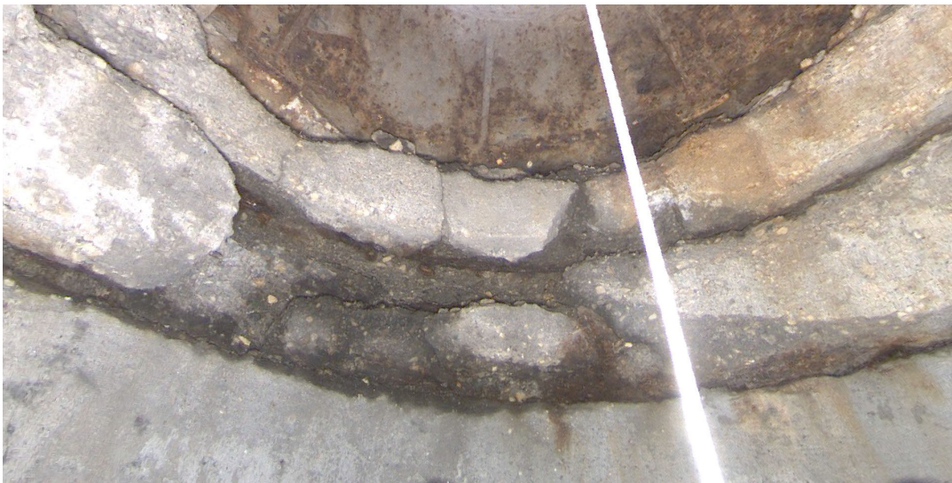
Photo #8 – (S-MH20011318) 0.48m deep - cracks present
