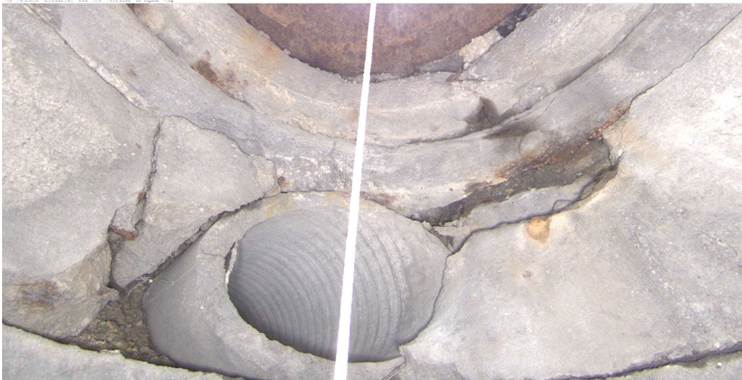
Photo #4 – (S-CB20011316) 0.24m-0.66m deep cracked adjuster ring, reducer, and broken riser
