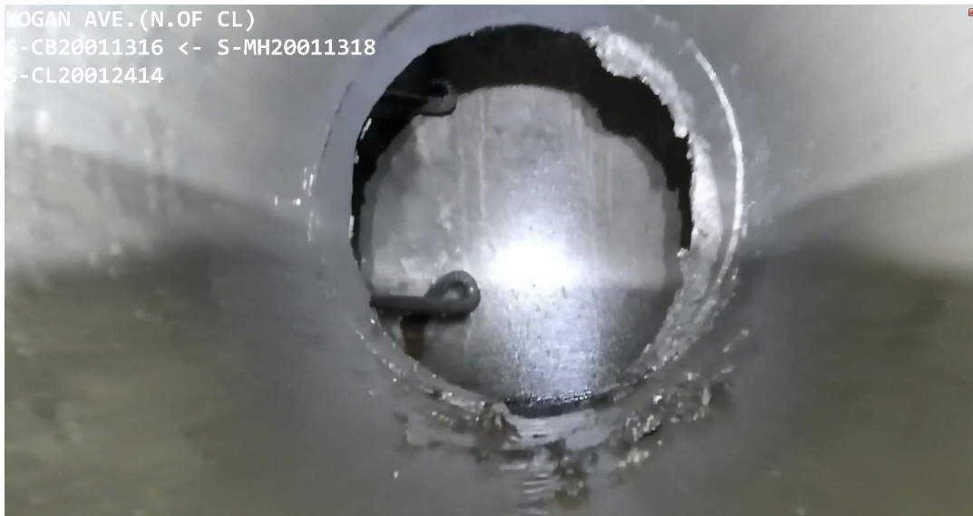
Photo #14 – (S-CL20012414) circumferential fracture from 5 o'clock to 7 o'clock 0.2m from CB
