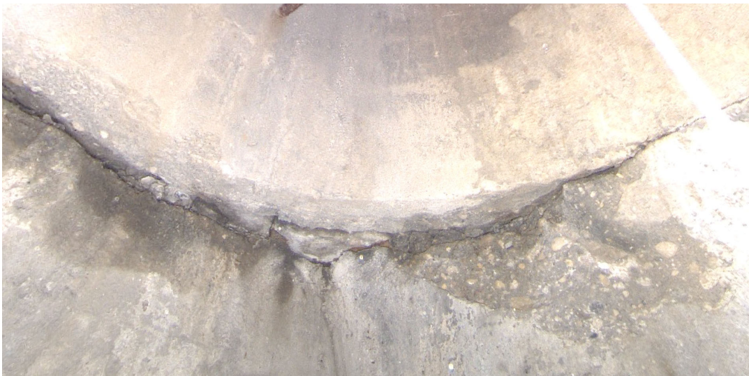
Photo #10 – (S-MH20011375) 0.81m deep - cracks/spalling underneath circular riser
