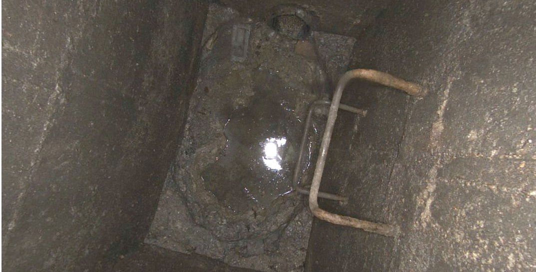
Photo #3 – (S-MH20011280) floor washed out
