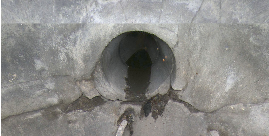
Photo #7 – (S-CB20011317) 0.7m deep - cracks present
