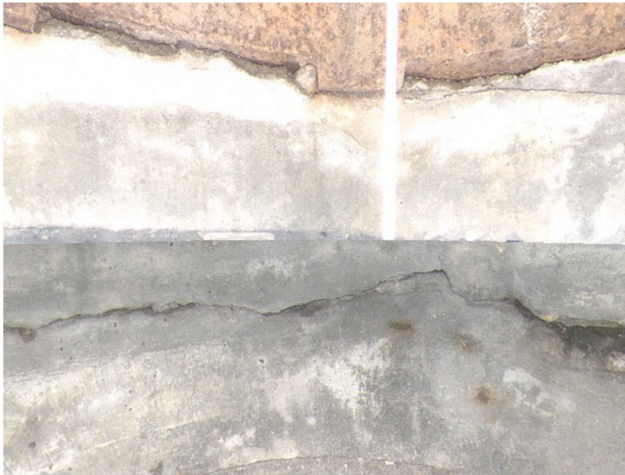
Photo #6 – (S-CB20011317) 0.48m deep - cracks present
