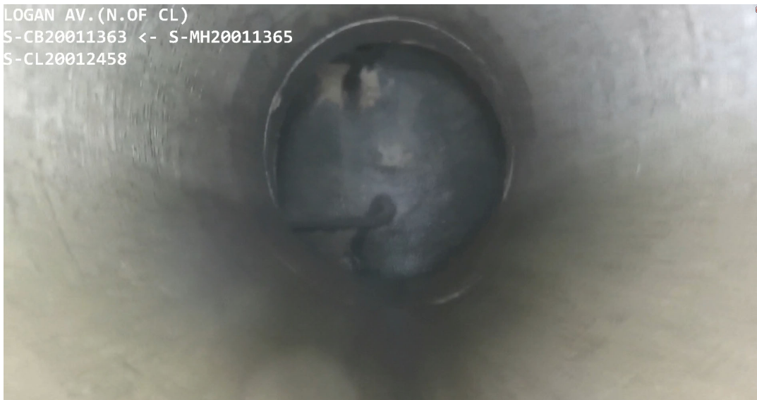
Photo #16 – (S-CL20012458) multiple circumferential cracks within 1.0m of catch basin
