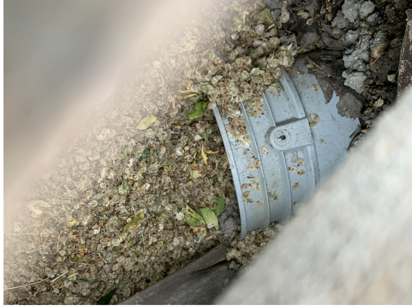
Photo #17 – (no asset number) catch pit connected to S-CB20011362 plastic pail instead of PVC pipe
