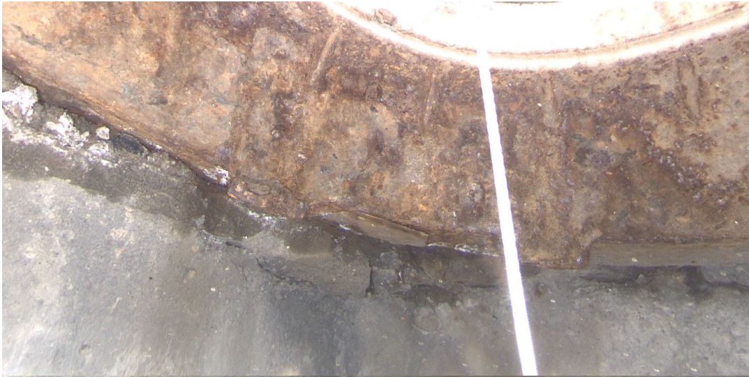
Photo #9 – (S-MH20011315) 0.15m deep - cracks/spalling present underneath frame
