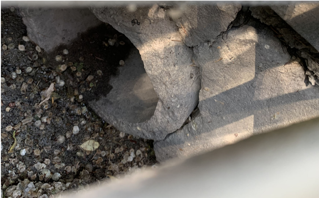
Photo #18 – (no asset number) catch pit connected to S-CB20011316 cracks around outlet
