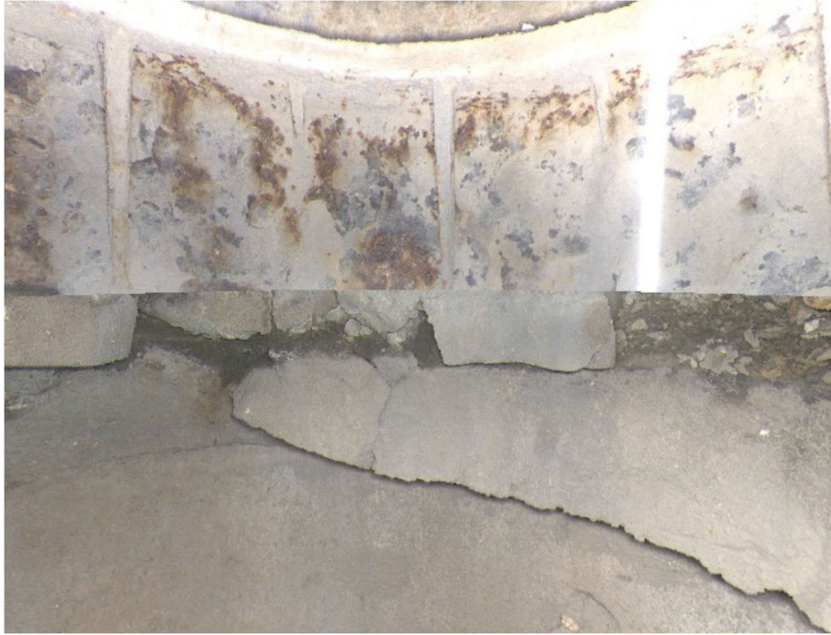
Photo #11 – (S-MH20011365) 0.27m-0.38m deep - cracks/spalling underneath frame and in 900mm-750mm reducer
