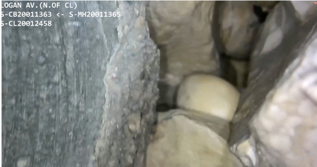
Photo #15 – (S-CL20012458) large void in pipe wall adjacent (within 0.3m) to manhole S-MH20011318
