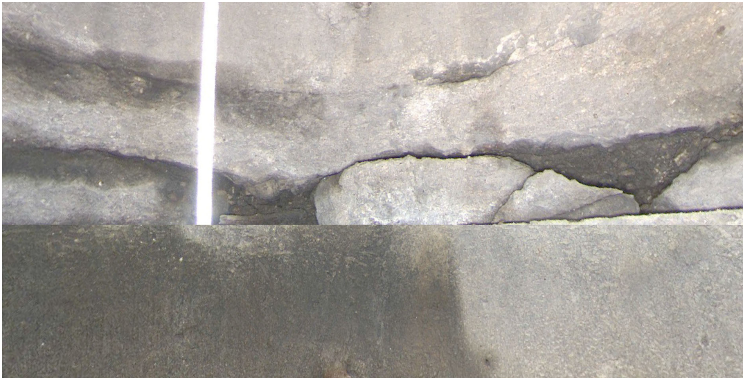
Photo #2 – (S-MH20011280) 0.58m deep multiple breaks throughout ring – soil visible
