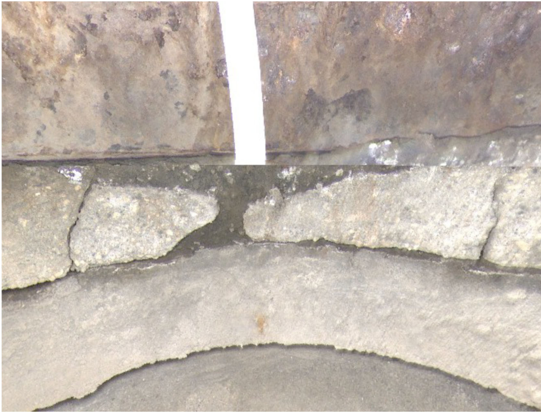
Photo #1 – (S-MH20011285) 0.28m deep multiple breaks throughout ring – soil visible
