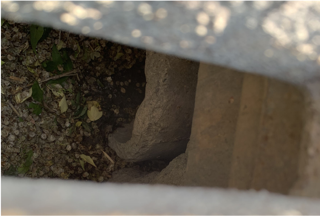
Photo #19 – (no asset number) catch pit connected to S-CB20011317 void around outlet pipe
