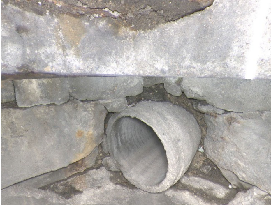
Photo #13 – (S-MH20011362) 0.25m-1.05m deep - multiple fractures in adjustment ring, reducer and riser – soil visible
