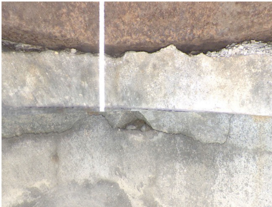
Photo #12 – (S-MH20011363) 0.18m-0.33m deep - cracks/spalling underneath frame and in 900mm-750mm reducer
