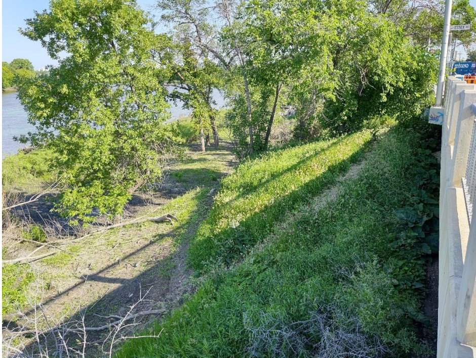
Photo 9: Looking downstream at the top of bank near the upstream edge of the project area (July 12, 2022)
