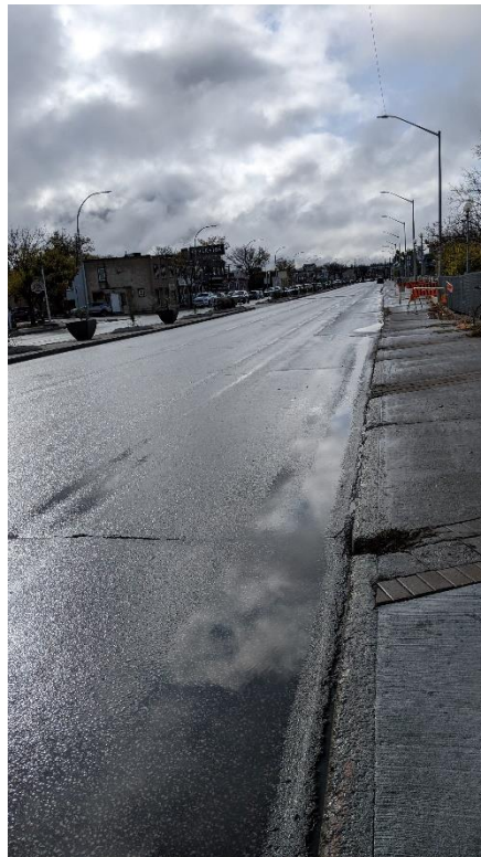
Photo 6: Looking south on St. Mary's at closed sidewalk segment after a rain event. CB at failure not low spot with ponding occurring in gutter (October 14, 2022)
