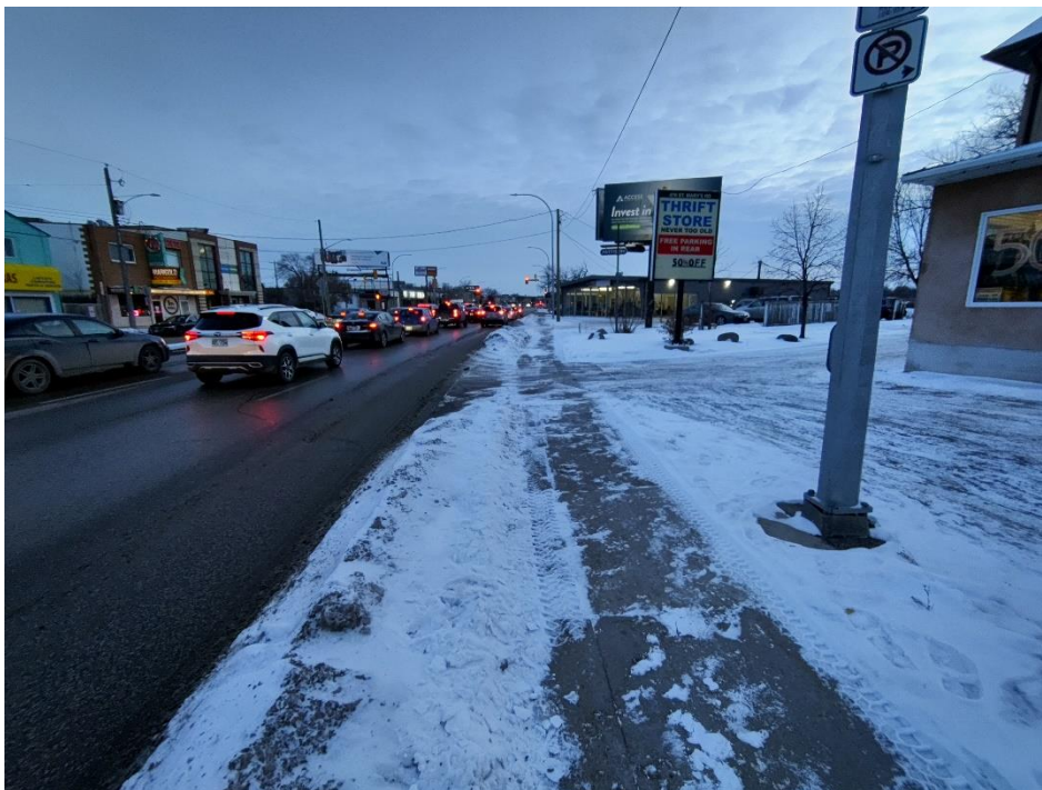
Photo 18: Looking south near top of construction access ramp. Caution must be exercised around existing signs and utilities (December 1, 2022)
