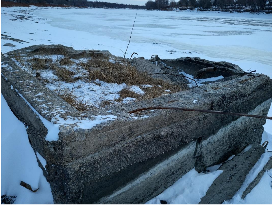
Photo 21: Old concrete block (to be removed) marks the downstream limit of riprap (refer to drawings for details). (December 1, 2022)
