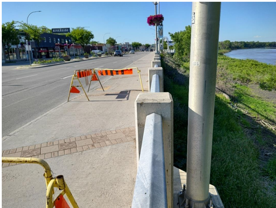
Photo 4: Looking upstream at the top of bank near the upstream edge of the project area (July 12, 2022)
