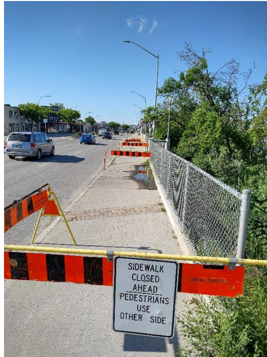
Photo 3: Looking south on St. Mary's at closed sidewalk segment (July 12, 2022)
