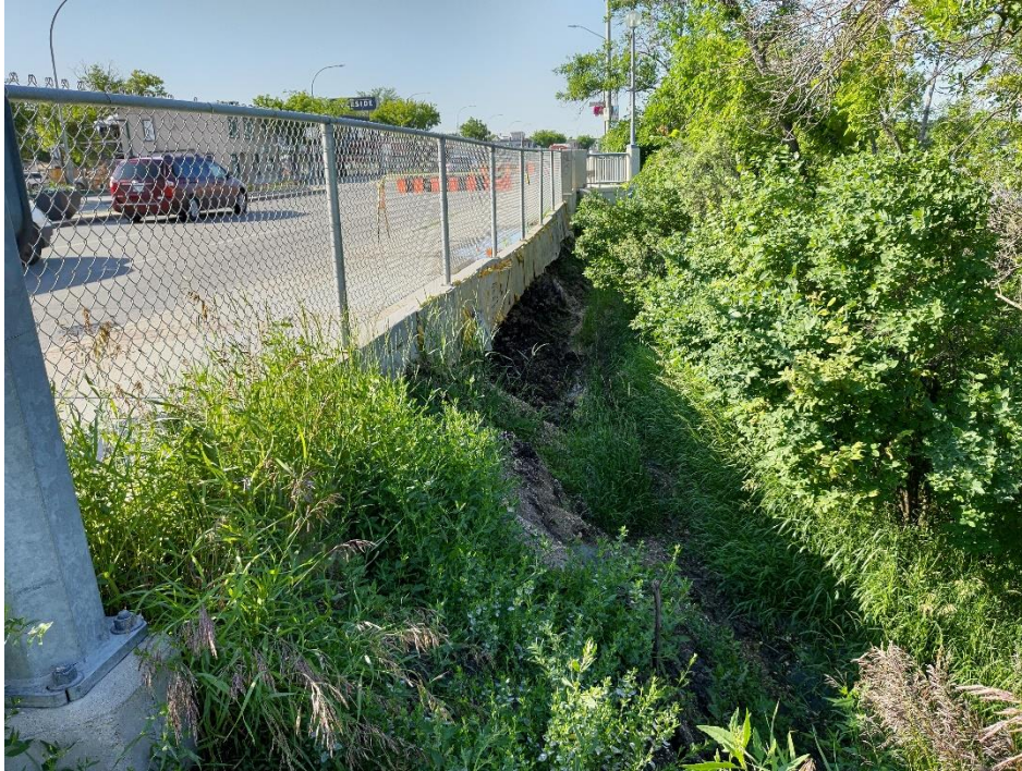
Photo 7: Looking south on St. Mary's at closed sidewalk segment. Significant undermining (July 12, 2022)
