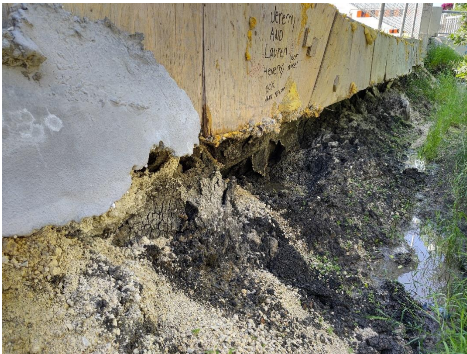
Photo 8: Close-up view of upper bank failure undercutting the sidewalk (July 12, 2022)
