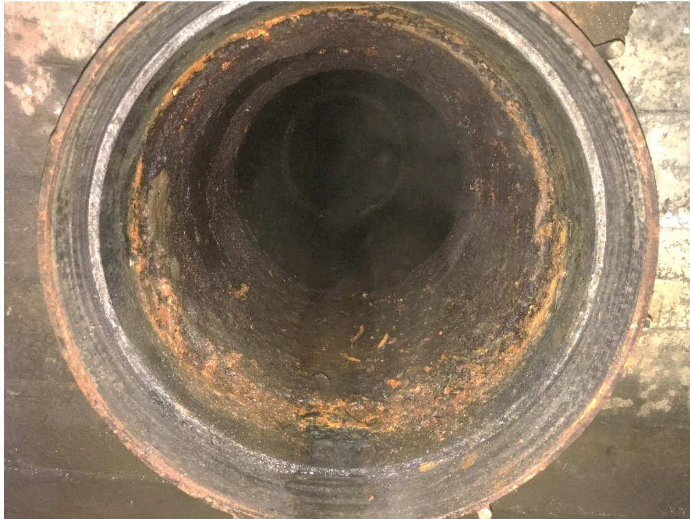
East Side - 600 feeder main (interior)
