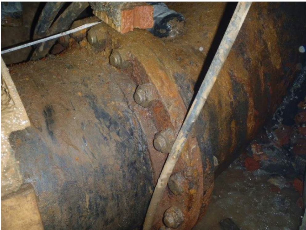
West Side – Existing 600 mm feeder main lower 90 deg bend lower flange connection
