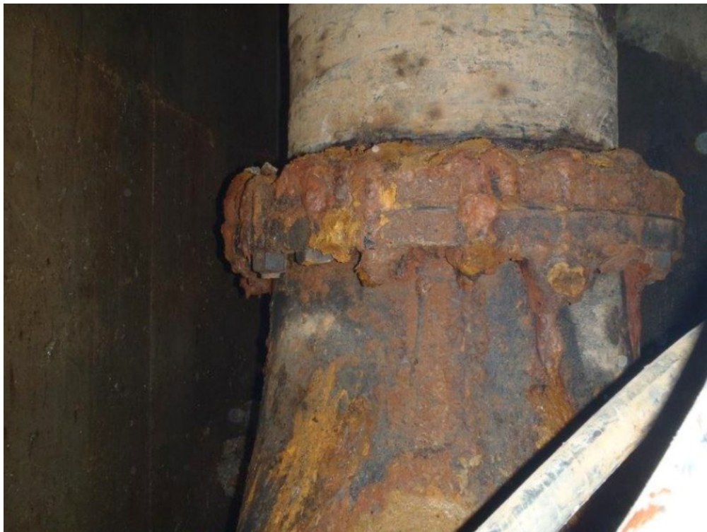
West Side – Existing 600 mm feeder main lower 90 deg bend upper flange connection
