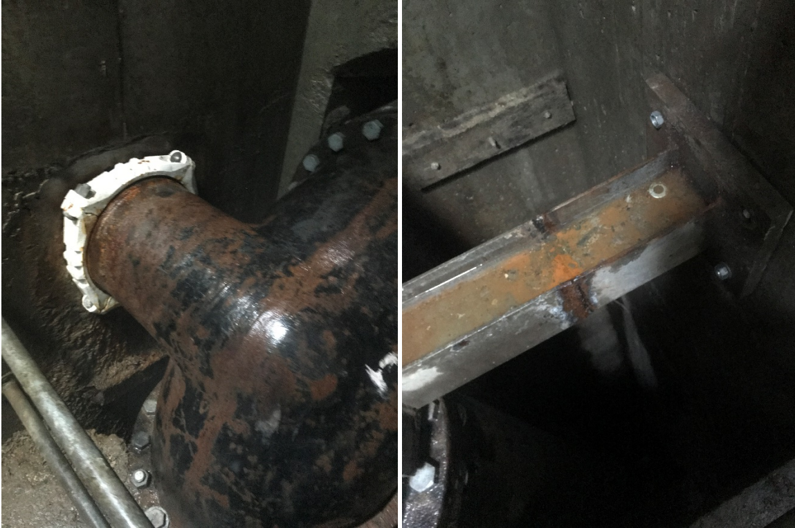
West Side – Existing tunnel shaft - Side-outlet elbow
