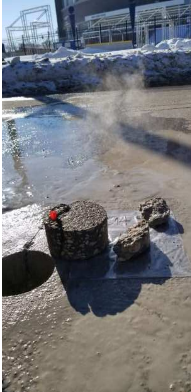
South bound transvers joint, Sta. 0+233. Could not extract concrete core due to crumbling
