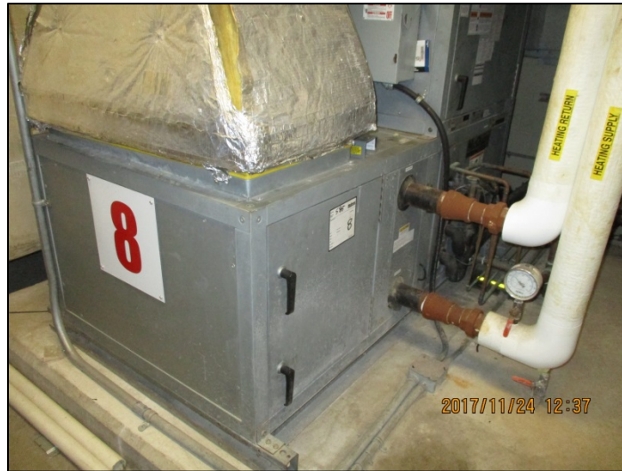
PHOTO 11 AIR HANDLING UNIT AH-8
