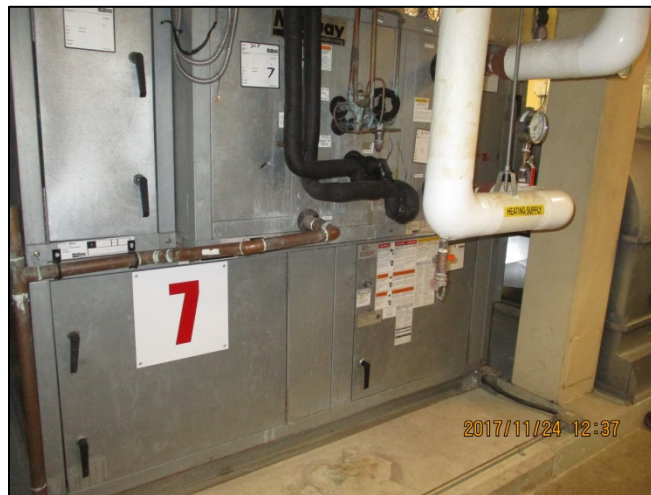
PHOTO 10 AIR HANDLING UNIT AH-7
