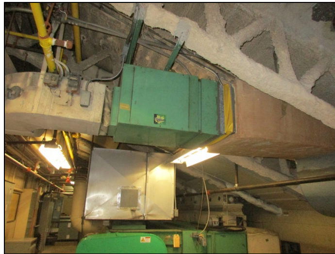
PHOTO 5 AIR HANDLING UNIT AH-5
