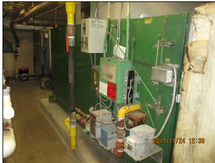
PHOTO 8 AIR HANDLING UNIT AH-1
