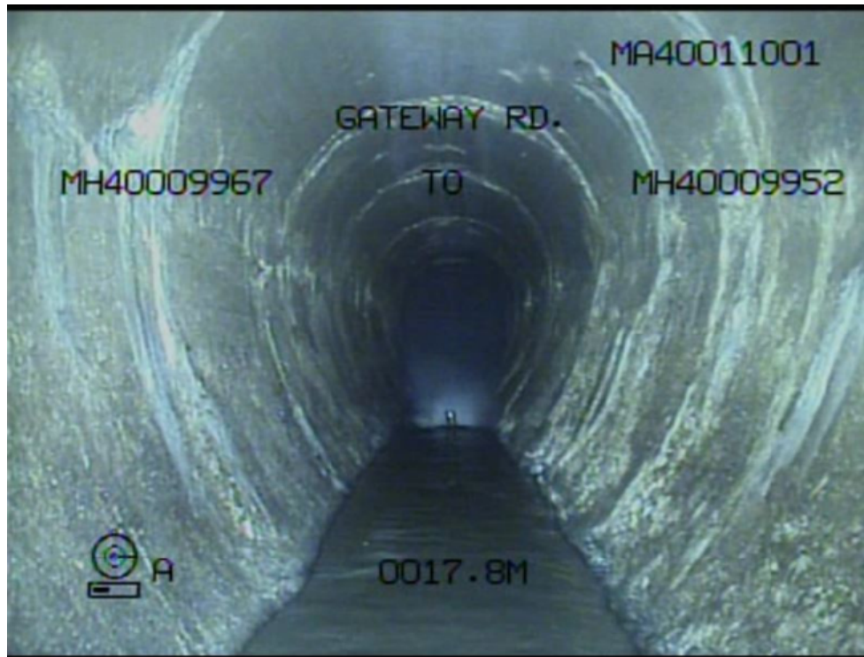
Figure 11: S-MA40011001 – Encrustation and Surface Spalling
