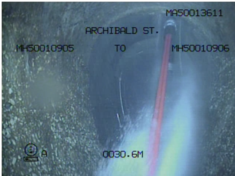
Figure 3: S-MA50013611 - Existing Liner at Downstream MH
