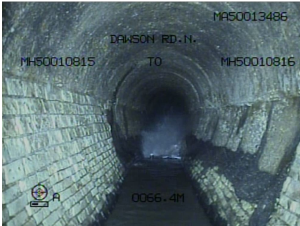
Figure 9: S-MA50013486 – Missing Bricks
