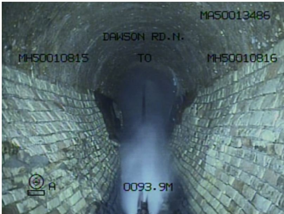
Figure 10: S-MA50013486 – Bulging Walls
