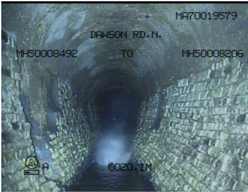
Figure 5: S-MA70019579 – Missing Bricks, Large Service
