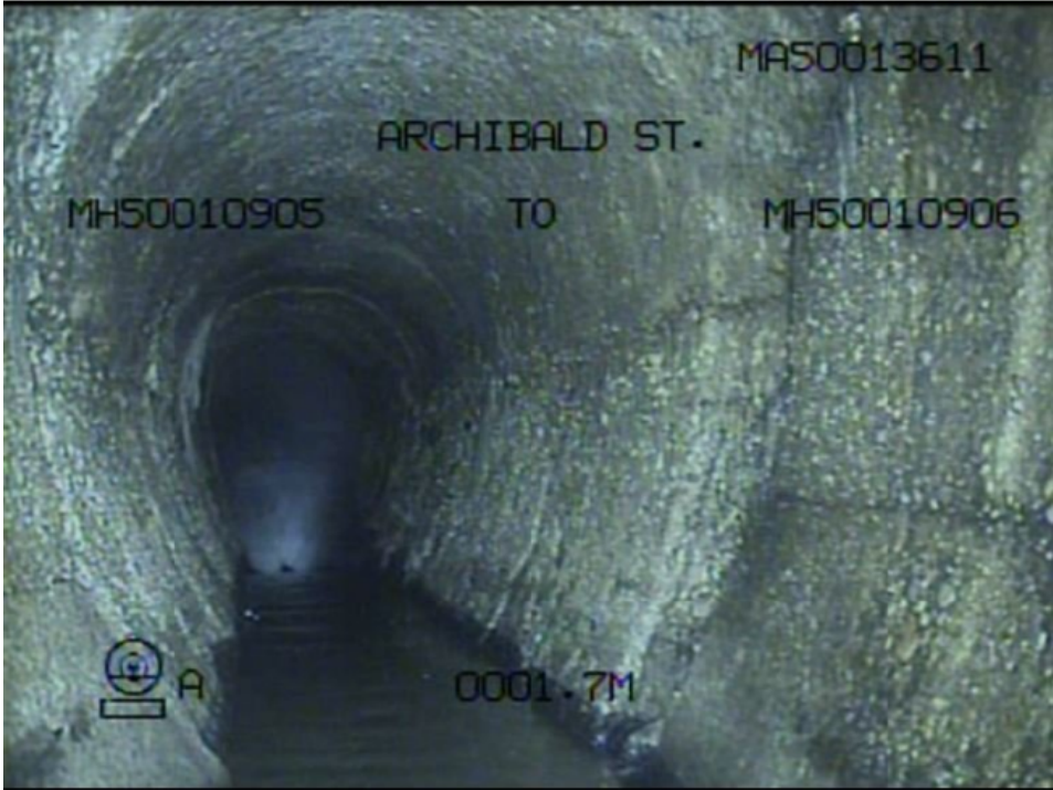
Figure 2: S-MA50013611 – Surface Spalling
