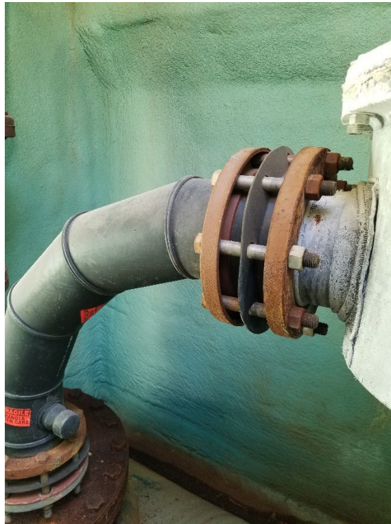
Photo 3 - ARC #6 (ID Unknown) Piping looking Northeast.
