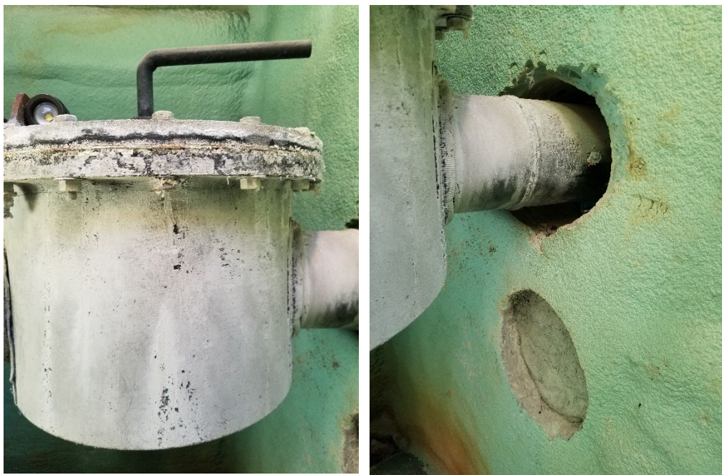
Photo 4 - ARC #6 (ID Unknown) Piping at Connection to Vent Piping at South Wall.
