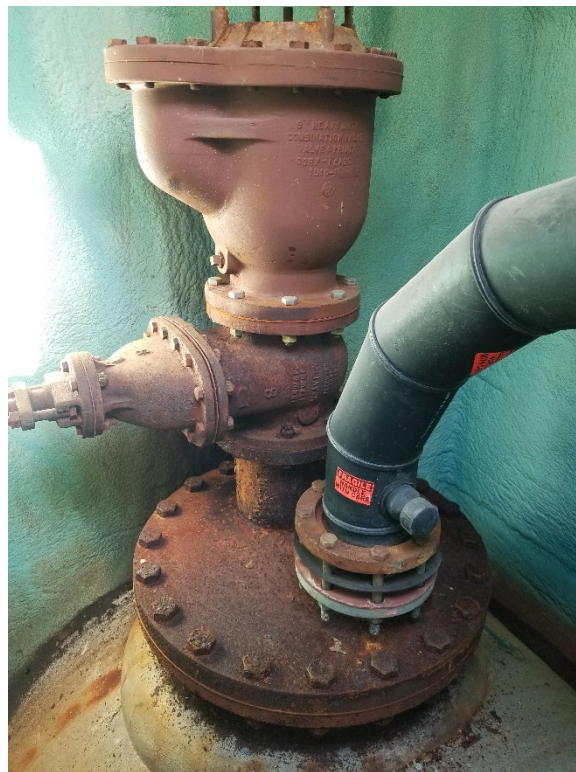
Photo 2 - ARC #6 (ID Unknown) Blind Flange and Piping, From Bottom of Ladder Access looking North.
