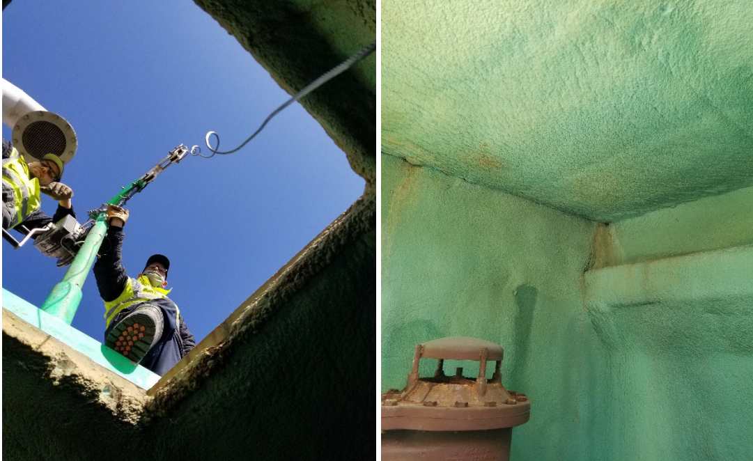
Photo 5 - ARC #6 (ID Unknown) General Access Hatch (Left) and Roof Slab (Right) from Top of Pipe at Ladder Access.
