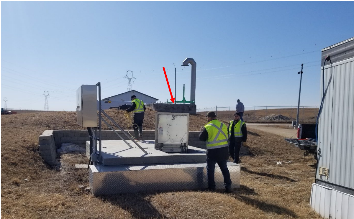
Photo 1 - Air Release Chamber (ARC) #6 (ID Unknown) at Water Treatment Plant Facility looking Southwest.
