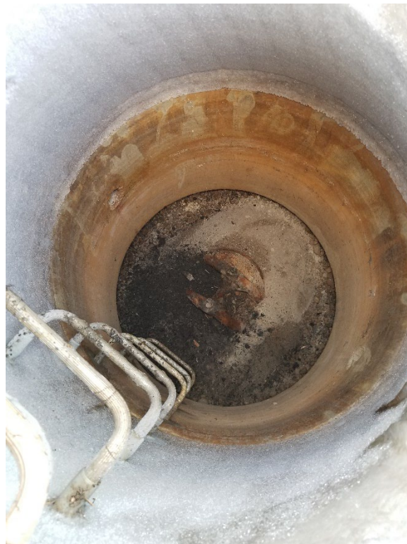
Photo 8 - Typical Pressure Manhole and Pressure Hatch from Grade.
