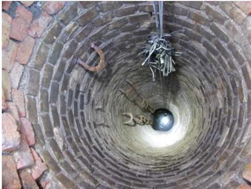
Metcalfe Wet Well
